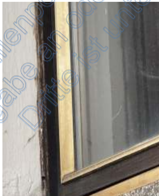
Detail veraltete Fenster
