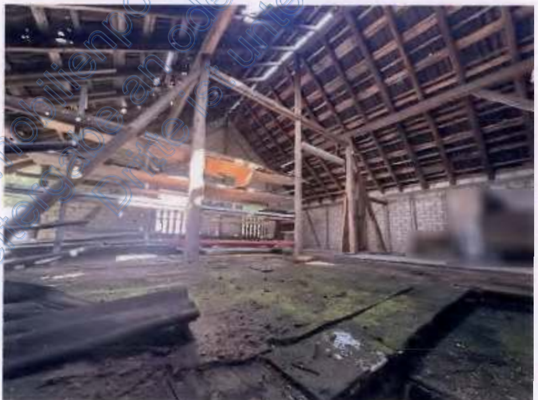
Speicher in Scheune DG
