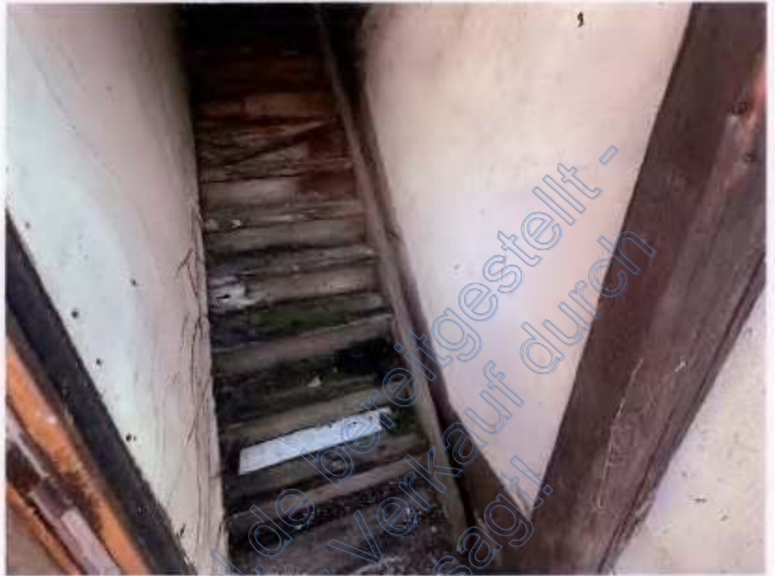
Treppe (marode) in Scheune zu DG
