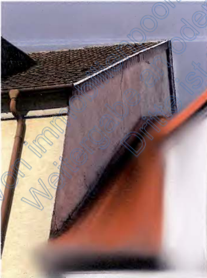
Detail Giebel; Riss
