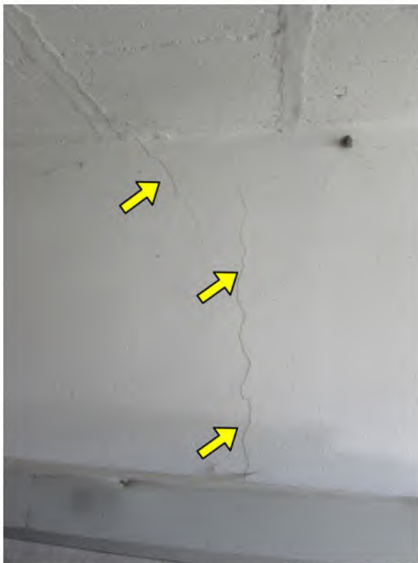
Foto 12: Erdgeschoss, Garage: Risse
