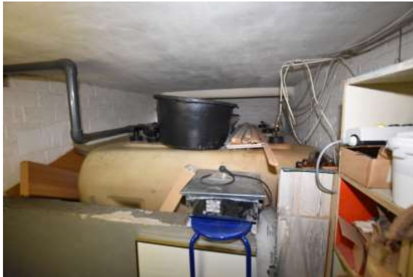
Öltanks in BT 2
