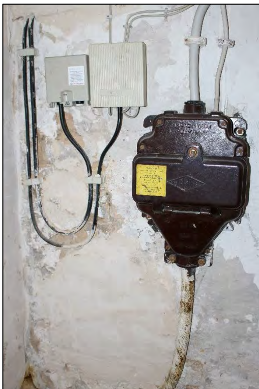
Foto Nr. 12: Kellergeschoss, Hausanschlüsse
