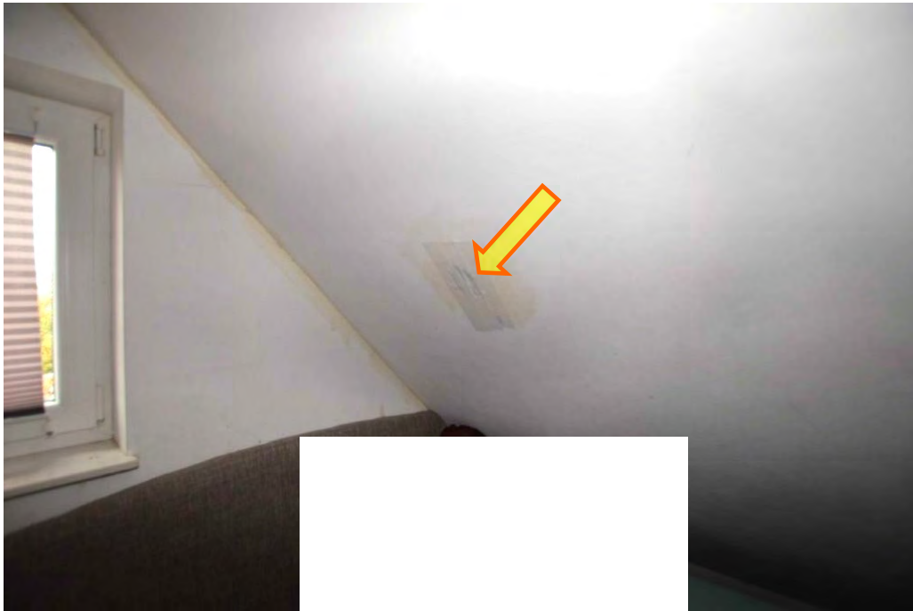
Spitzboden – Loch in Gipskartonplatte
