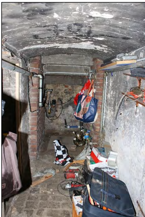
Foto Nr. 18: Kellergeschoss, Hausanschlüsse
