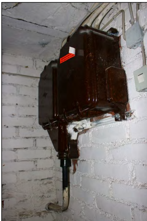
Foto Nr. 14: Kellergeschoss, Hausanschlüsse
