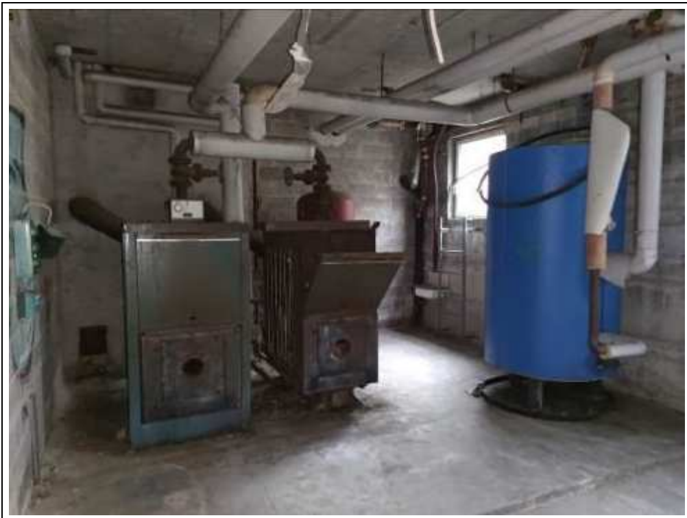
Blick in den Heizraum
