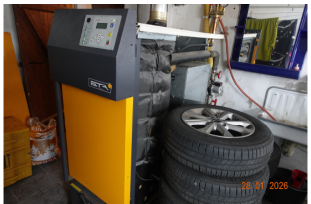
Pelletheizung in KG
