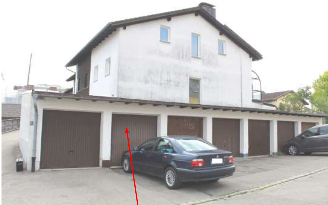
Abb. 5: FlNr. 868/15 – Garage, rissiger Asphaltbelag
