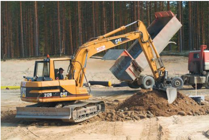
Figure 16.7 A hydraulic machine in action
