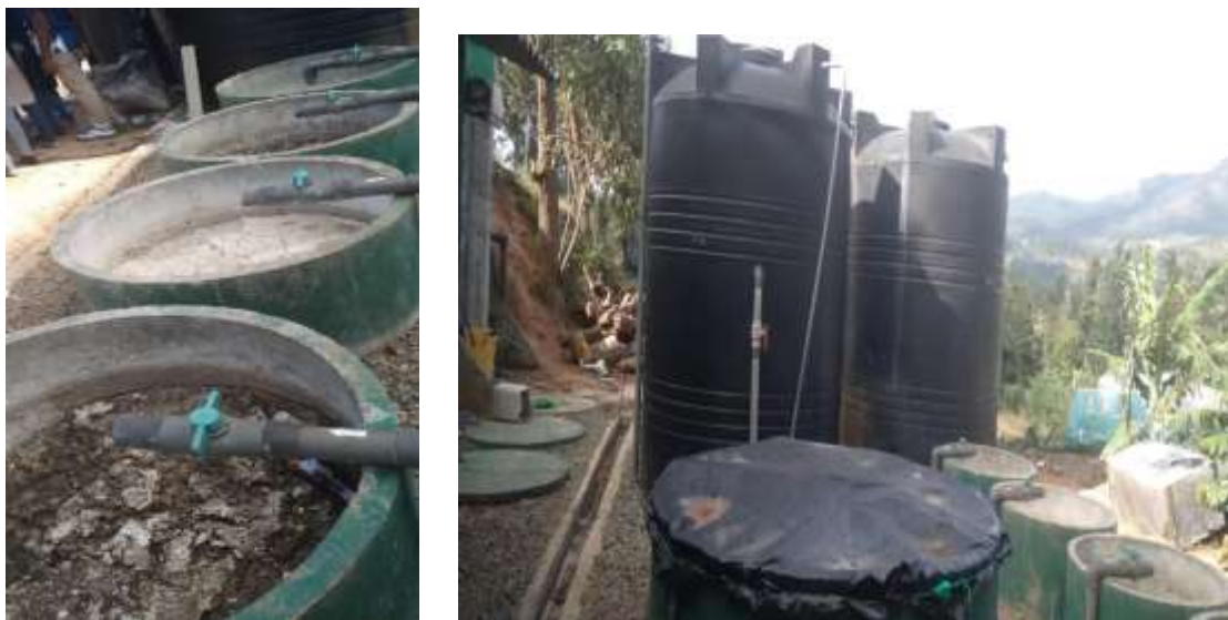
Figure 37: Major units of the Wastewater plant
