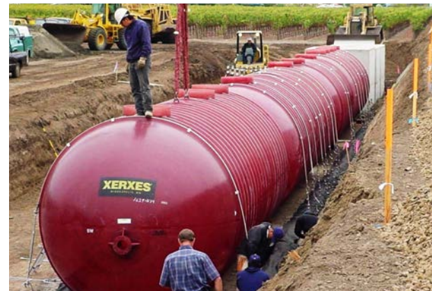
Underground metal cistern
