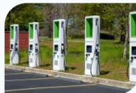
EV- Charging Station
