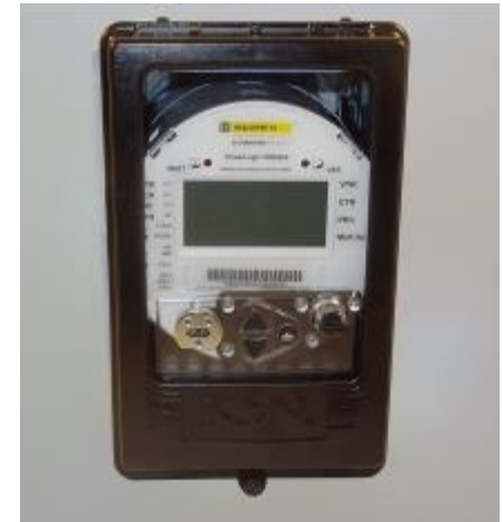
ION 8650 Retrofitted into Westinghouse/ABB cutout
