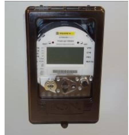
ION 8650 Retrofitted into Westinghouse/ABB cutout
