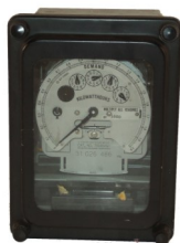
1. GE Meter in Panel
