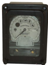
1. GE Meter in Panel
