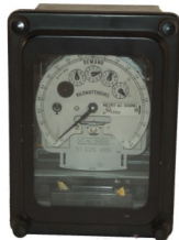
1. GE Meter in Panel
