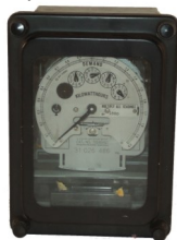
1. Old Meter in Panel
