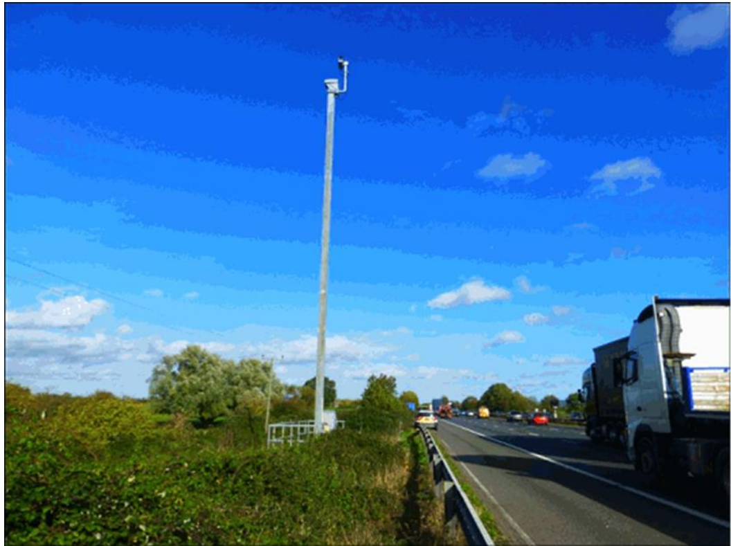
Figure 3-11 View of CCTV Mast 00041 Looking North
