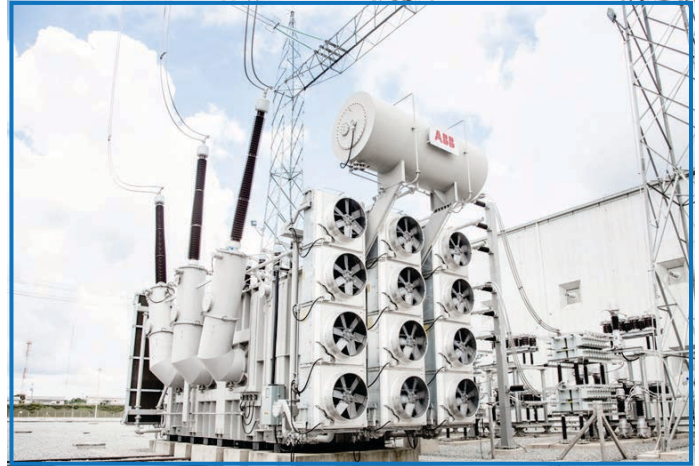
CONVERTER STATION TRANSFORMER
