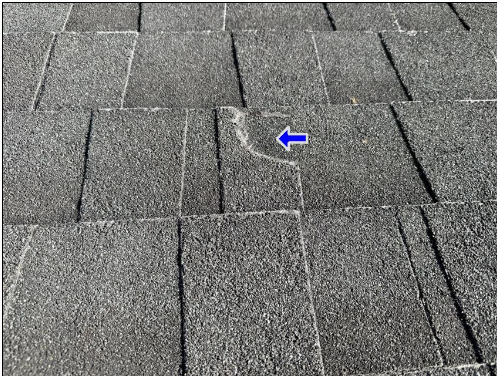
10.0 Item 1(Picture) worn/torn roof shingle
