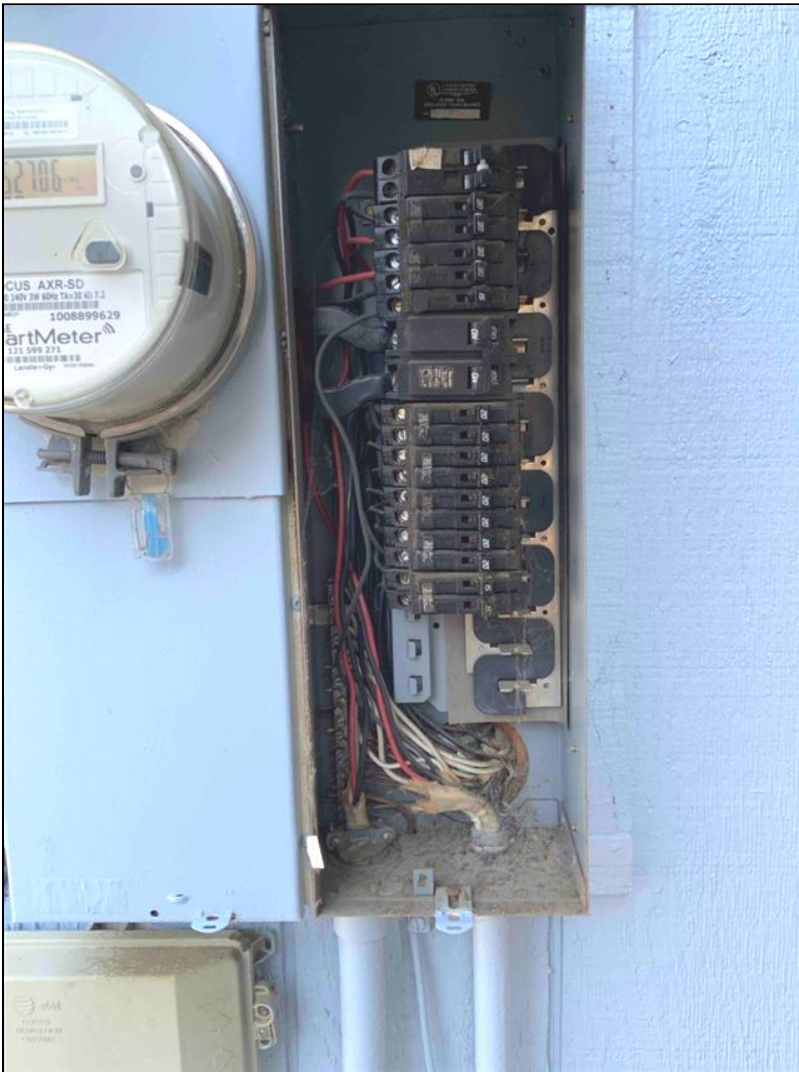
1.1 Item 1(Picture) All in one electrical panel
