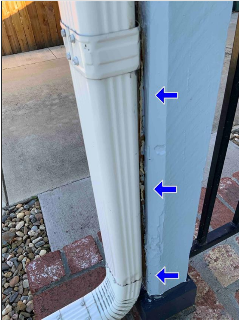
2.3 Item 3(Picture) damage to the front porch support post.
