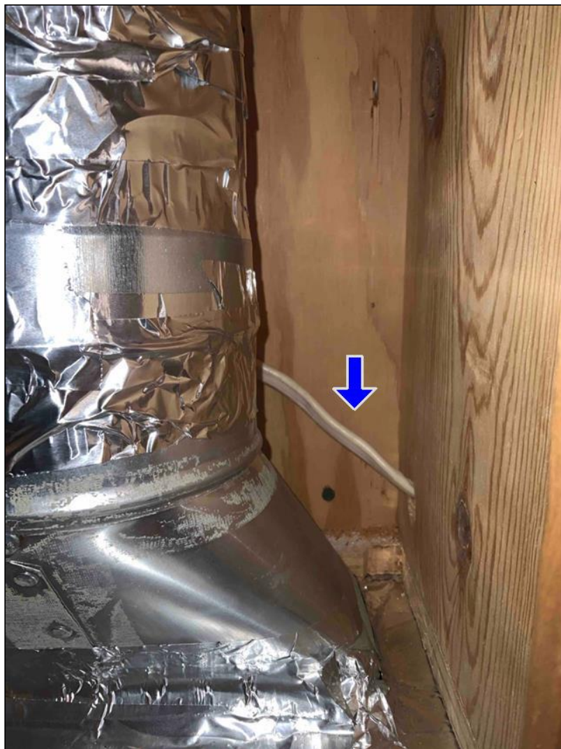
1.3 Item 1(Picture) exposed wire in the kitchen cabinet above the stove fan
