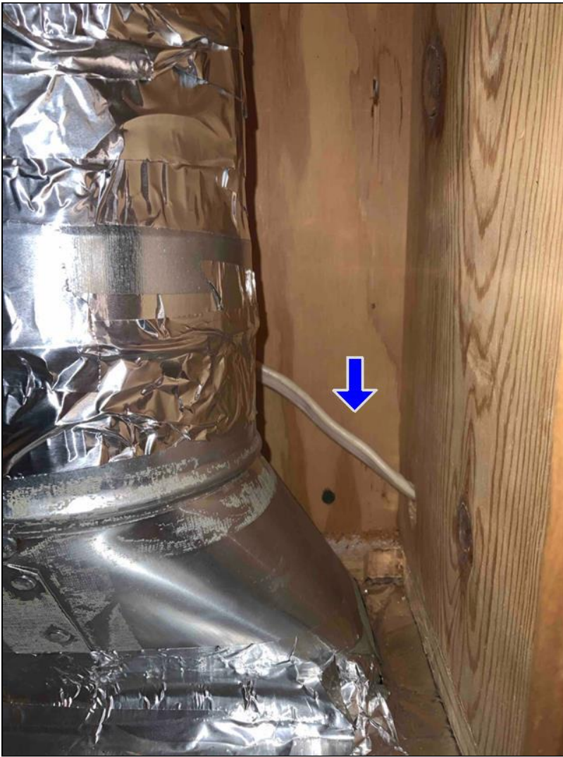
1.3 Item 1(Picture) exposed wire in the kitchen cabinet above the stove fan
