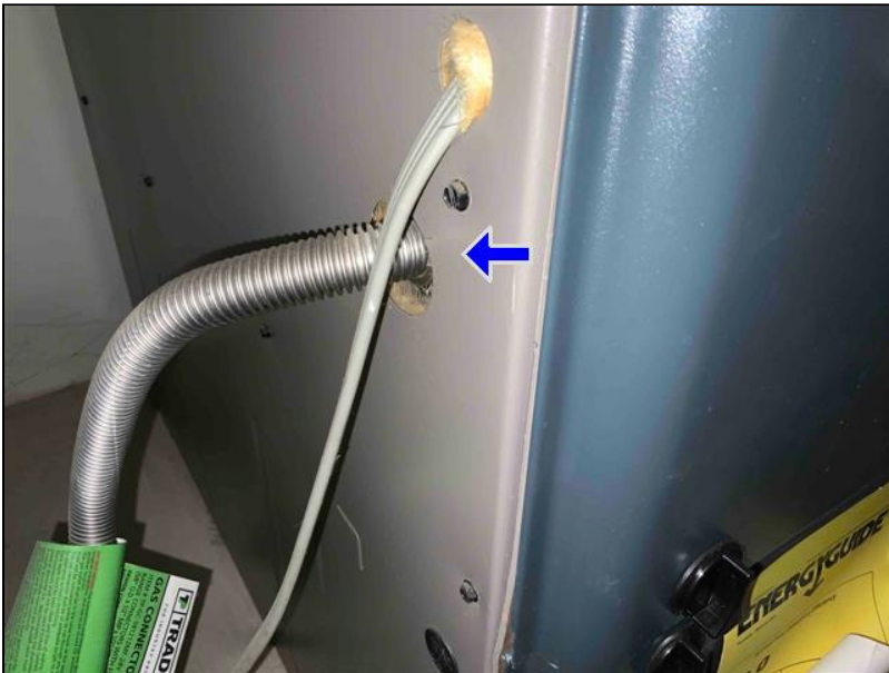
8.0 Item 1(Picture) gas supply line for the furnace enters through the sheet metal siding.
