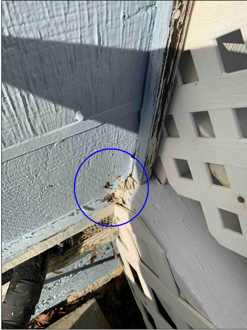
2.0 Item 1(Picture) Wood trim and siding damaged
