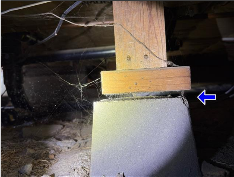
9.2 Item 1(Picture) support posts are not properly secured to the concrete piers
