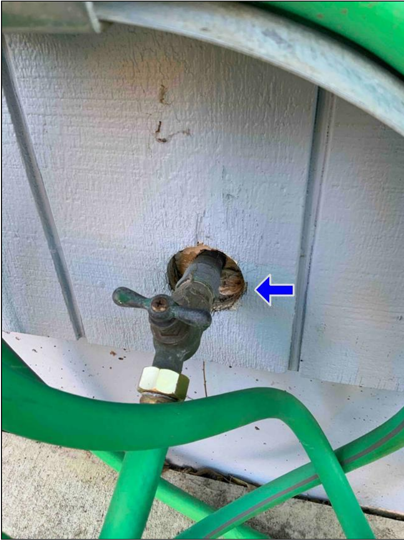
2.0 Item 2(Picture) holes/gaps to the siding
