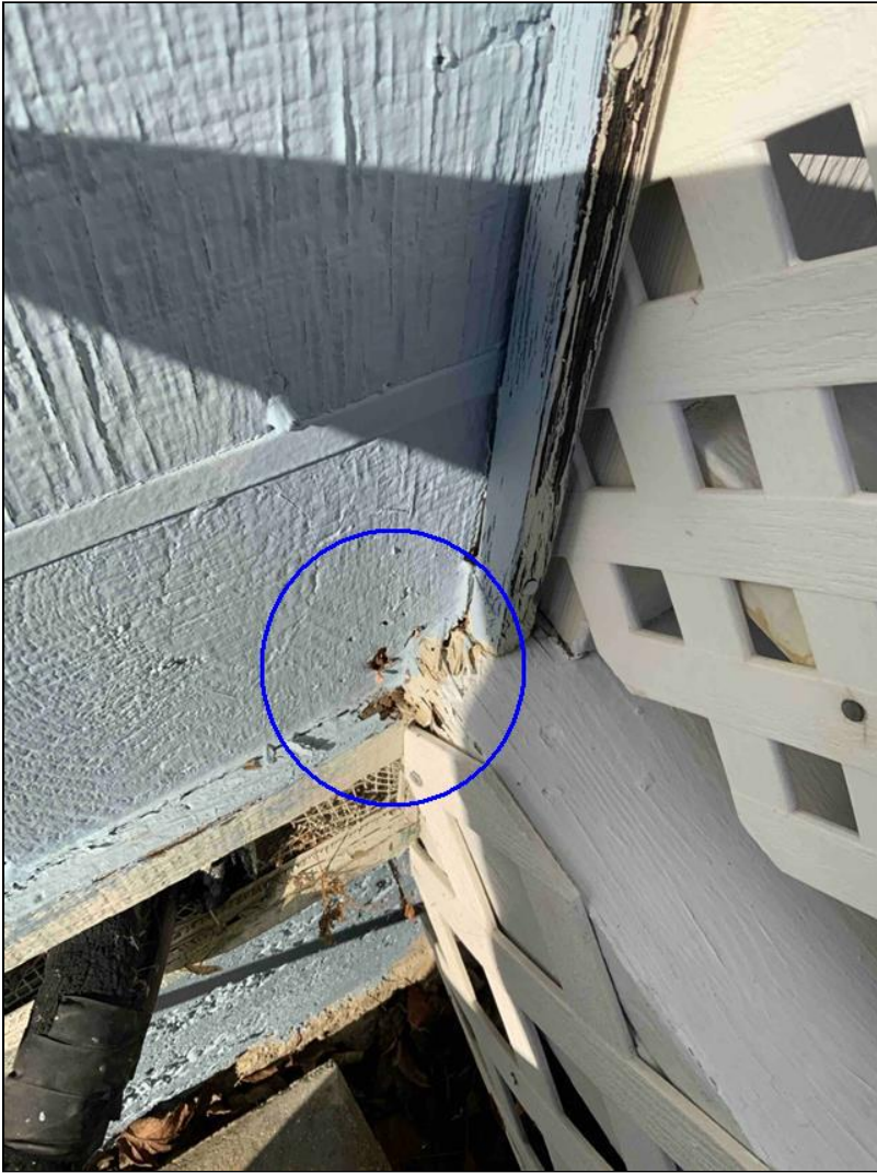
2.0 Item 1(Picture) Wood trim and siding damaged
