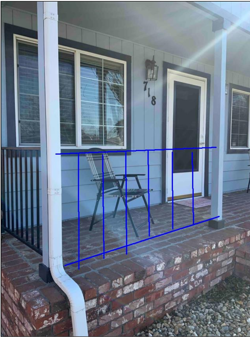
2.3 Item 1(Picture) recommends installing a railing system at the front walkway/porch area for additional safety
