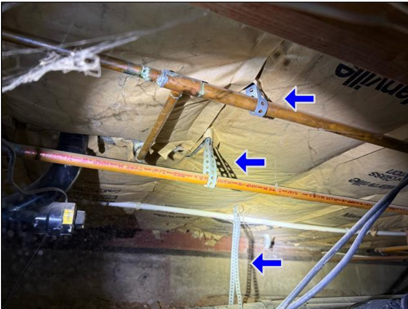
7.1 Item 1(Picture) type of material used for the plumbing straps for the water supply lines in the crawl space appears to be the incorrect type used
