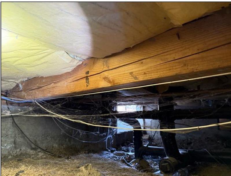
9.3 Item 1(Picture) cracks to some of the main support girder beams in the crawl space
