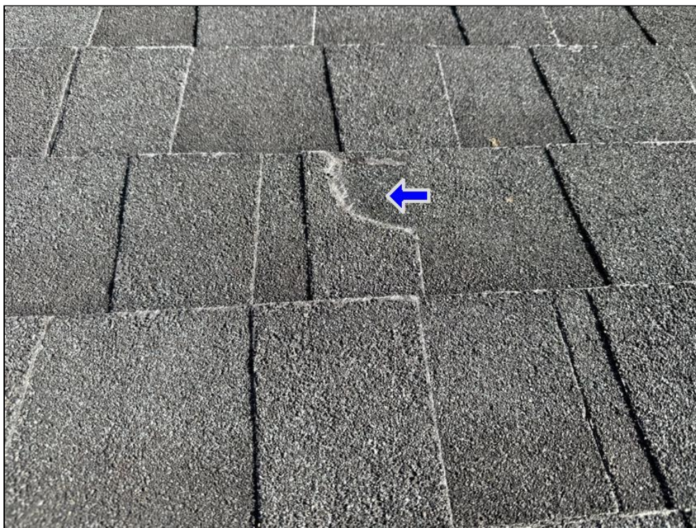
10.0 Item 1(Picture) worn/torn roof shingle
