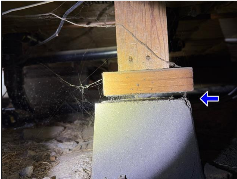
9.2 Item 1(Picture) support posts are not properly secured to the concrete piers
