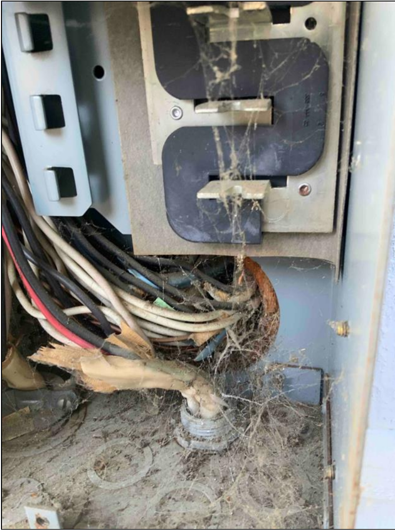
1.1 Item 2(Picture) missing wire clamp at the rear of the electrical main panel.
