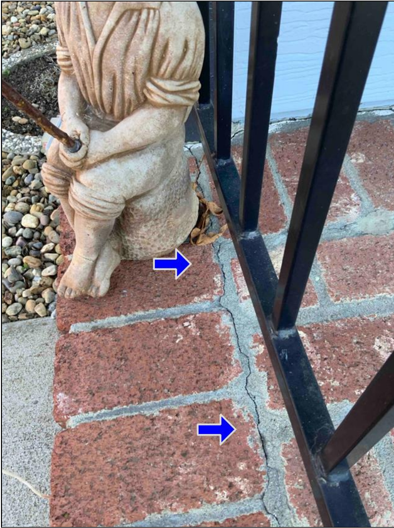
2.3 Item 2(Picture) cracks in the front porch brick mortar
