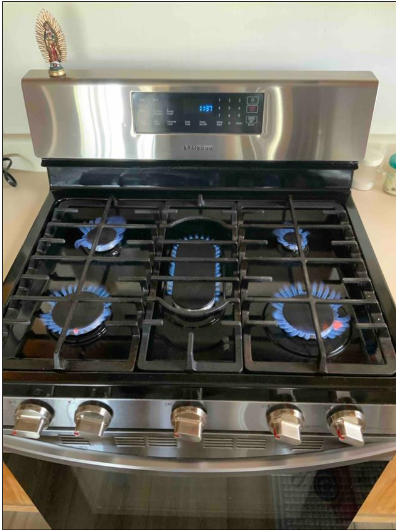
4.1 Item 1(Picture) Stove top operating
