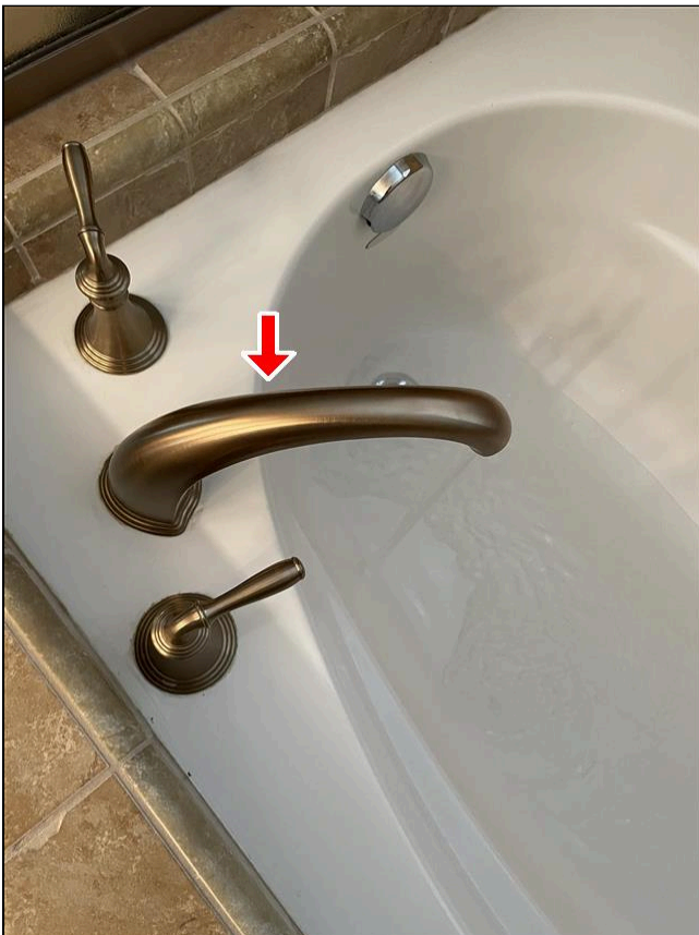
6.3 Item 1(Picture) master tub spout loose
