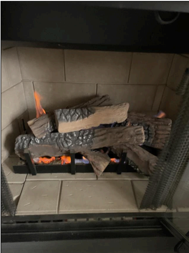
8.5 Item 1(Picture) fireplace functional
