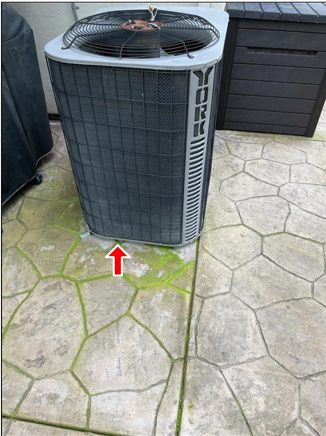
8.3 Item 1(Picture) air unit should be on pad
