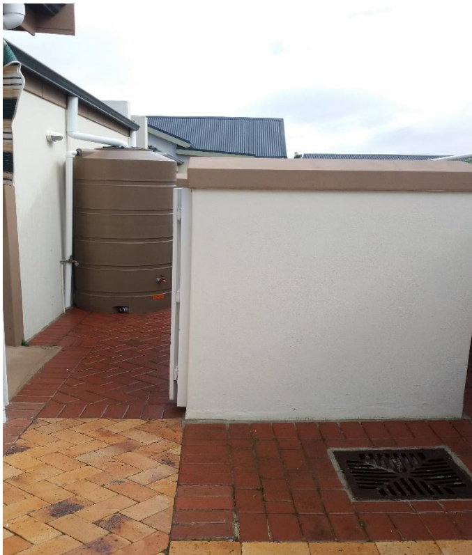
Photo 33 - example of 1000 litre installed in Courtyard – unit 91 (Exclusive Use Area) – post consent at AGM or SGM (Photo taken before the tank was painted)
