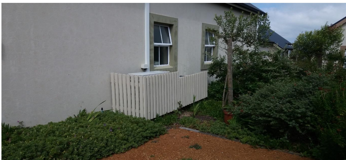
Photo 29 – Specified Heat pump and air conditioner enclosure
