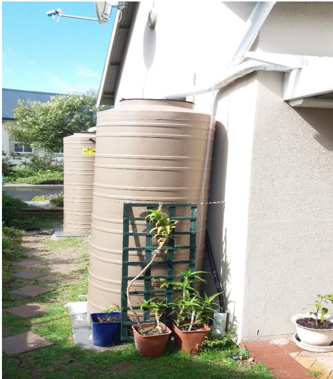
Photo 32 - unit 138 Example of two x 1000 litre tanks and permitted changes to downpipes (Photo taken before painting of tank/cladding)
