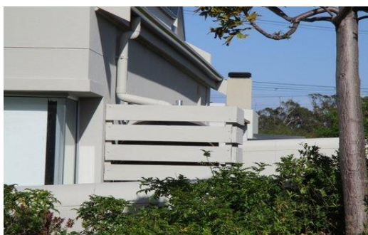
Photo 31 of tank installation enclosed - permitted wood panels and permitted changes to down pipes
