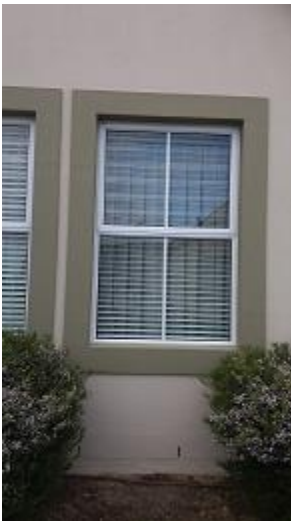
Photo 23 - Unit 88 - Clear burglar bars
