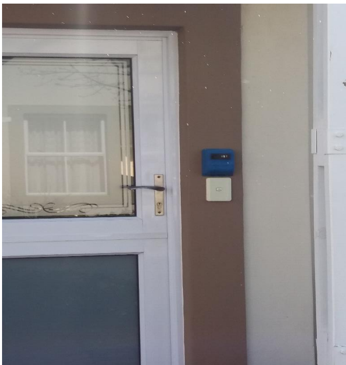
Photo 34 Example of Key Safe installed at front door
