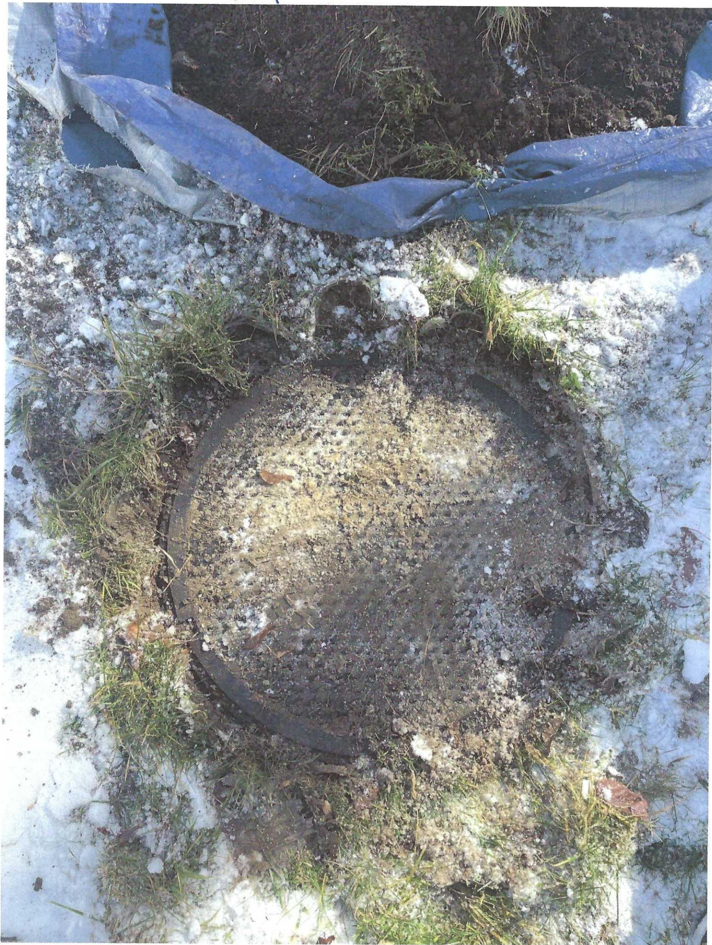
Pump chamber cover
