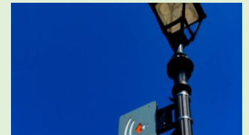
Smart Street Lighting Scheduled light timings to provide right level of lighting
