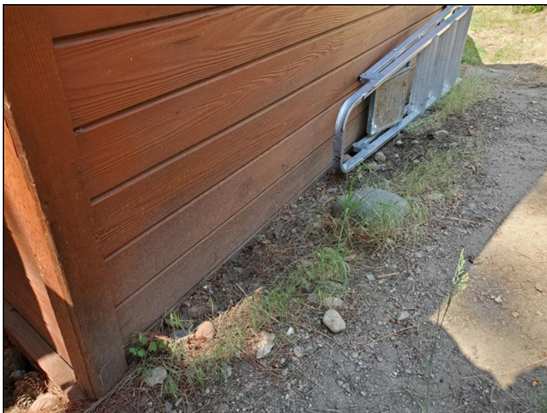
2.0 Item 1(Picture) Earth to wood contact
