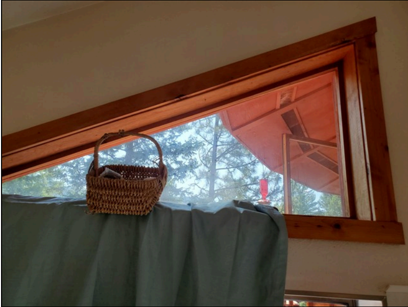
3.6 Item 1(Picture) Cloudy window in upstairs bathroom
