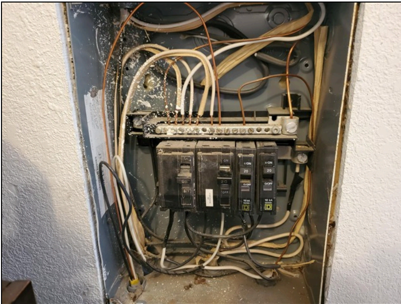
6.1 Item 2(Picture) Cabin sub panel- neutrals/grounds bonded
