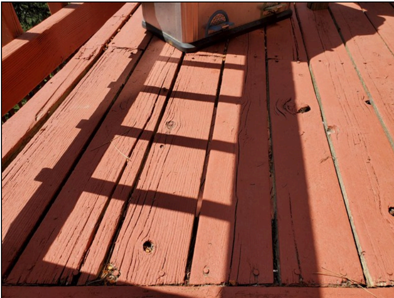
2.3 Item 3(Picture) Decay
