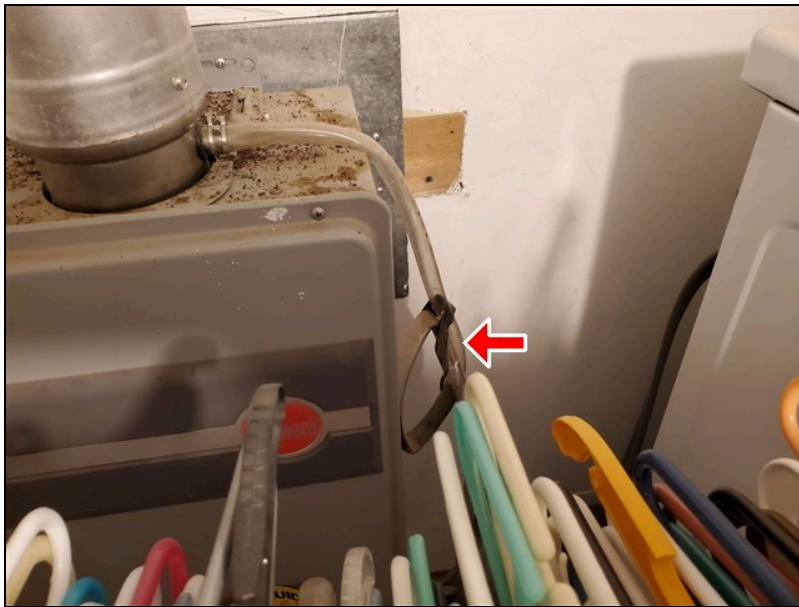
5.2 Item 1(Picture) condensate drain blocked
