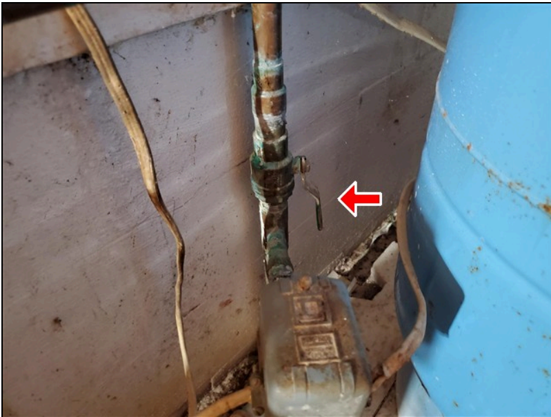
5.3 Item 2(Picture) Main water shut off valve
