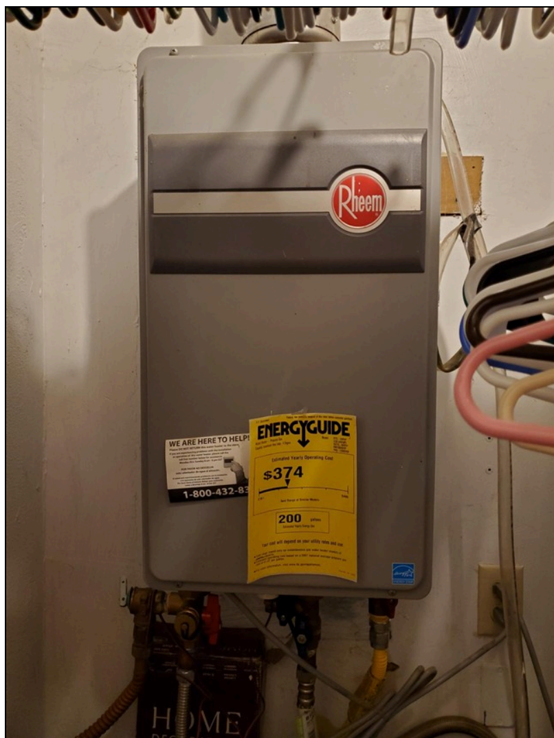
5.2 Item 2(Picture) Water heater
