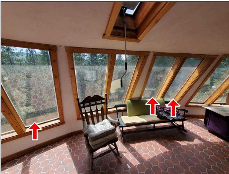
3.6 Item 3(Picture) Cloudy windows in sunroom
