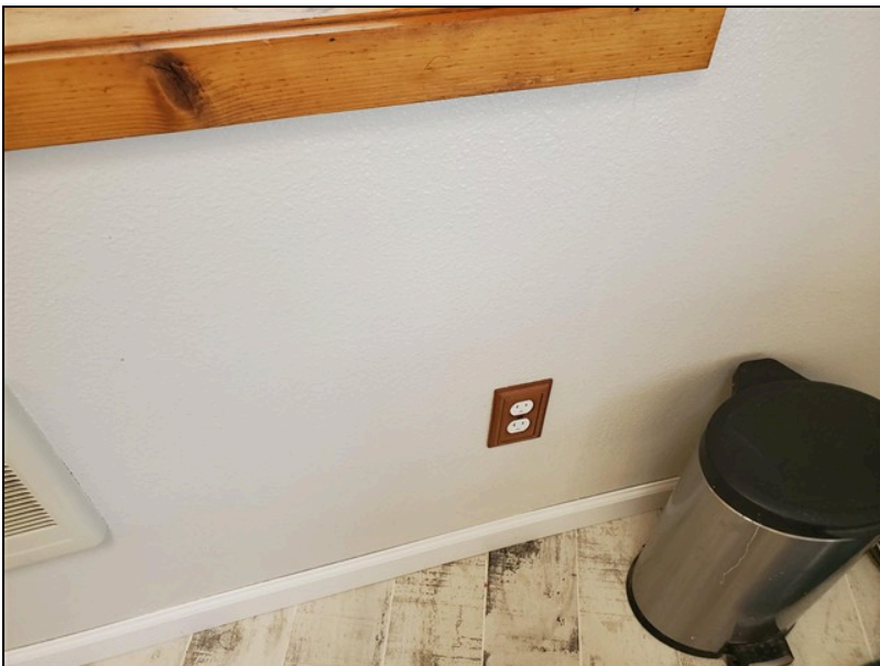
6.5 Item 1(Picture) Not GFCI protected
