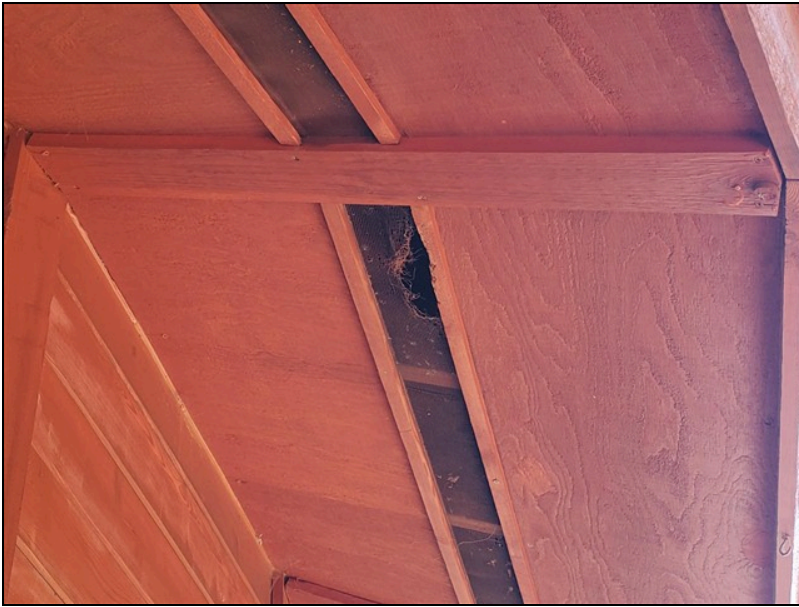
8.3 Item 1(Picture) hole in soffit vent
