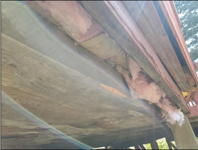
8.1 Item 2(Picture) gaps under sunroom
