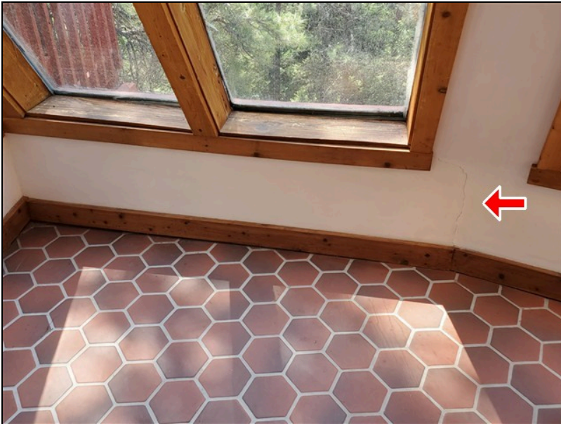
4.2 Item 2(Picture) cracks
