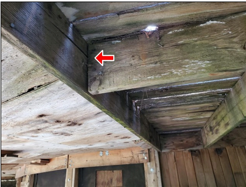
2.3 Item 7(Picture) connection loose
