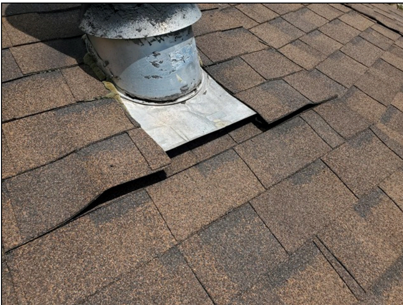
1.1 Item 1(Picture) loose flashing
