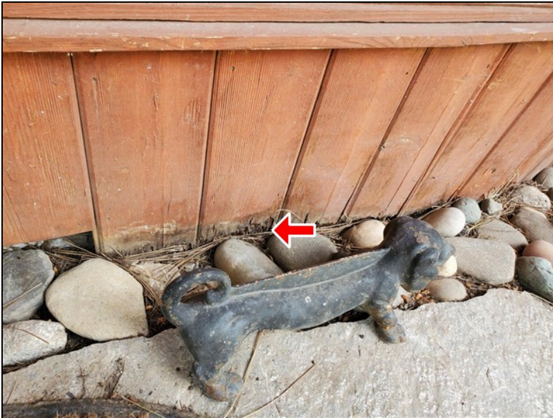
2.0 Item 2(Picture) Minor decay on skirt boards
