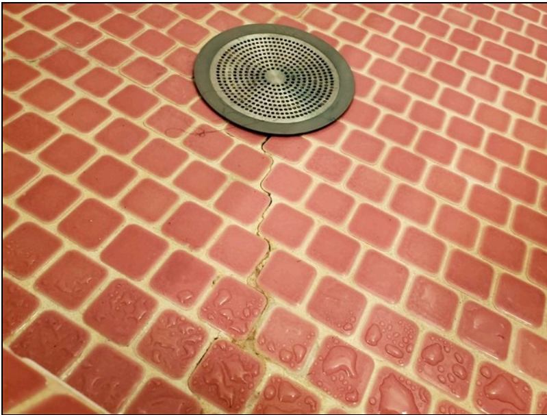
3.2 Item 1(Picture) Cracked grout
