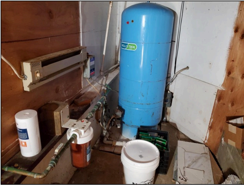
5.3 Item 1(Picture) Well equipment
