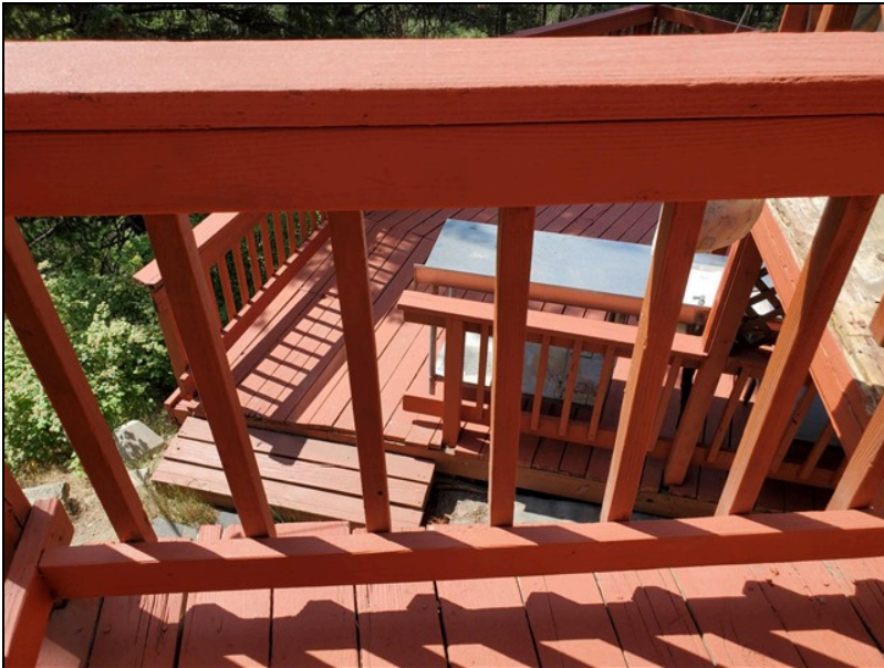
2.3 Item 2(Picture) Rail openings larger than 4" unsafe for children
