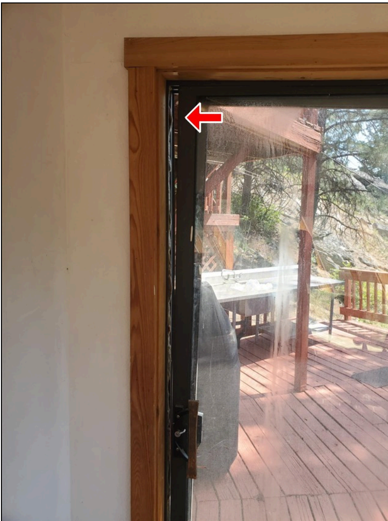
4.2 Item 3(Picture) doorway not square
