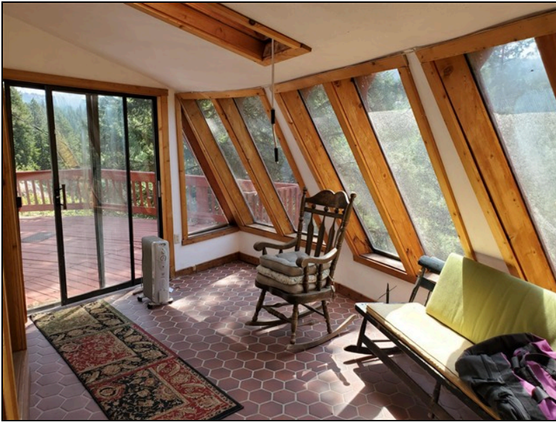
4.2 Item 1(Picture) Signs of settlement- Floor slopes
