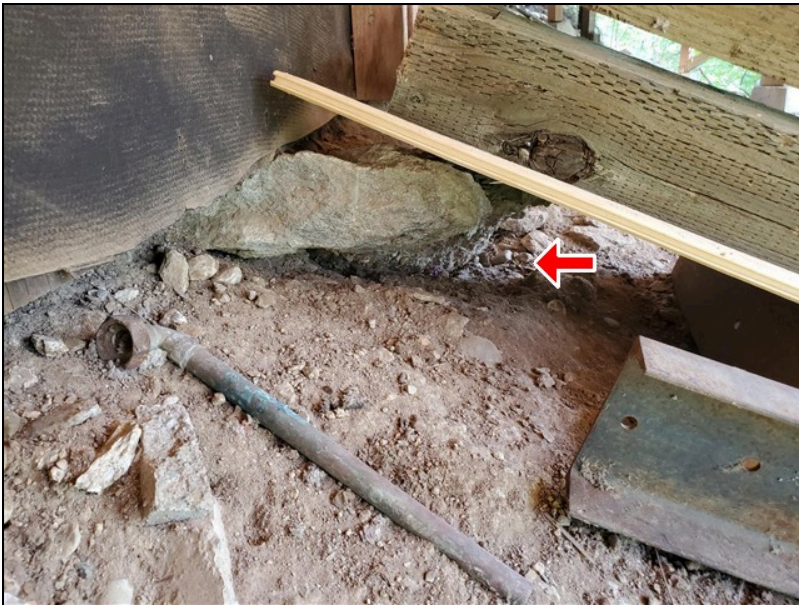
4.2 Item 5(Picture) erosion below pier
