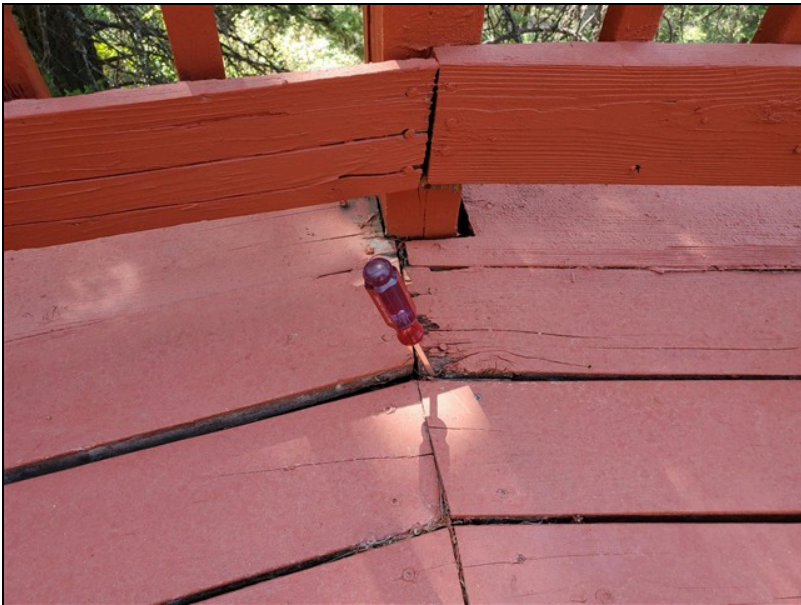
2.3 Item 5(Picture) decay
