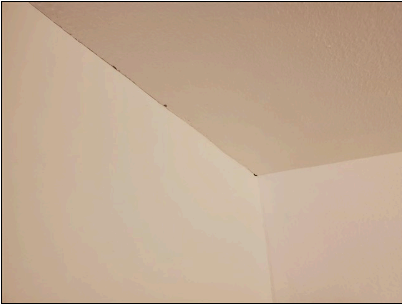
3.1 Item 1(Picture) crack
