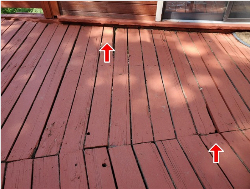
2.3 Item 6(Picture) deck decay
