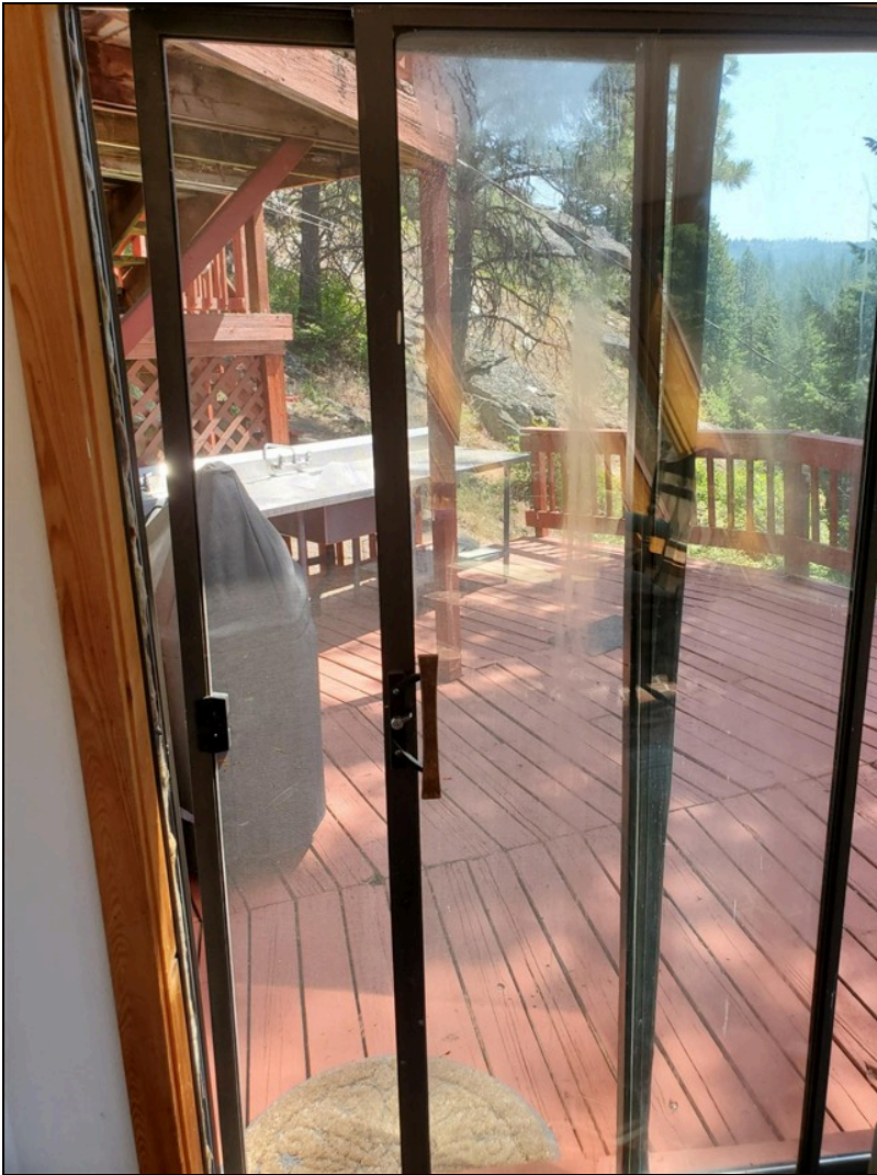
2.1 Item 1(Picture) Cloudy window in door
