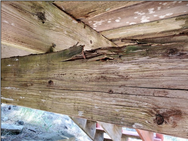
2.3 Item 4(Picture) decay
