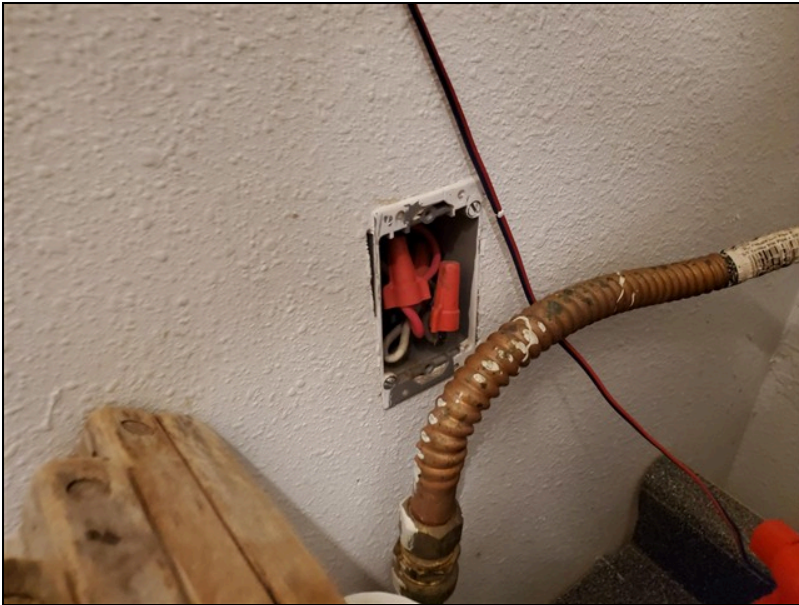
6.3 Item 1(Picture) Missing cover plate
