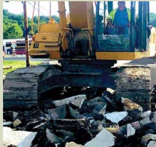
Shane Todisman working for Gershenson on the bridge replacement over Saline Creek on Hwy, a MODot project.
