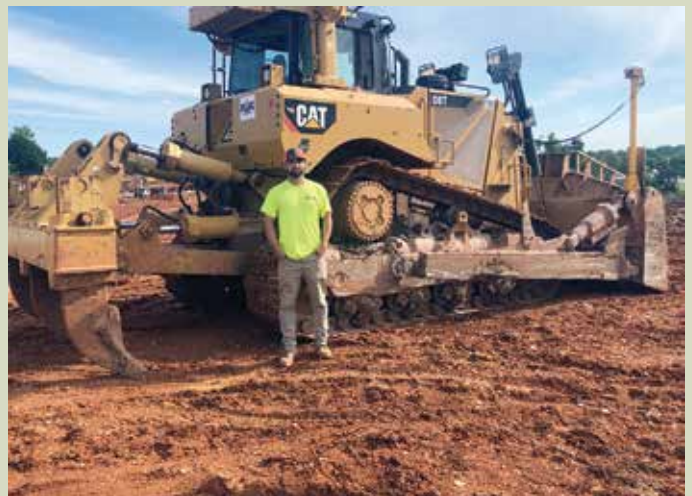
Tyler Slinkard working for R&K Excavation at the new Sugar Creek Apartments off of Hwy.
