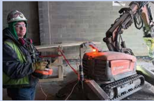
Austin Pieper running a remote control breaker at the Post Dispatch bldg .
