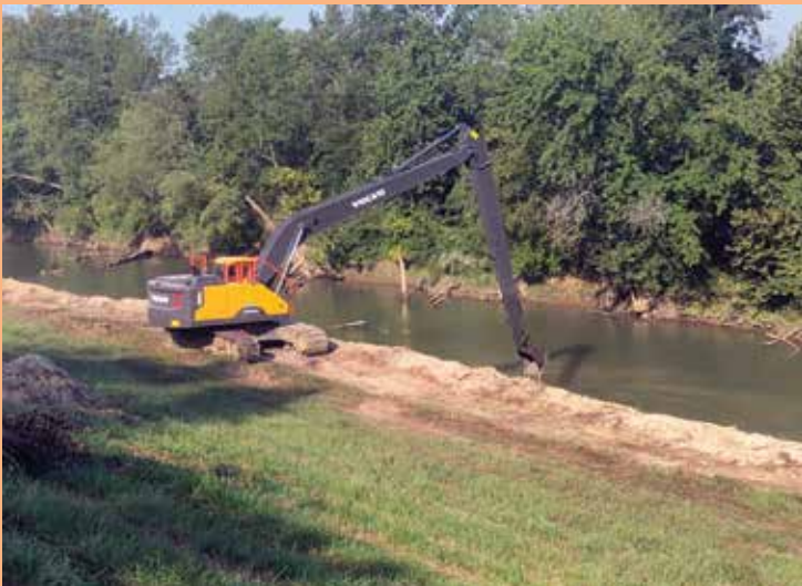
Rick Dennis placing rip rap for Bloomsdale Excavating on the Diversion Channel Job outside of Delta, Mo.
