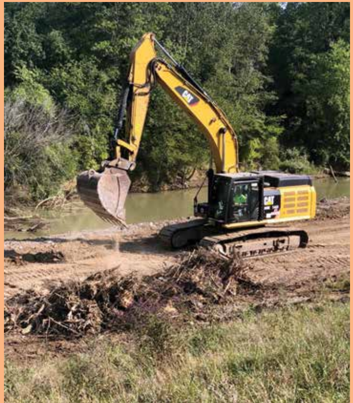
Kelly Shelby fixing slides and placing rip rap for Bloomsdale Excavating on the Diversion Channel Job outside of Delta, MO.
