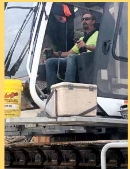
Walsh Construction at the Merchants Bridge. Operator-Michael Vaughn, not in photo apprentice Codey Brookman getting seat time. Good job.
