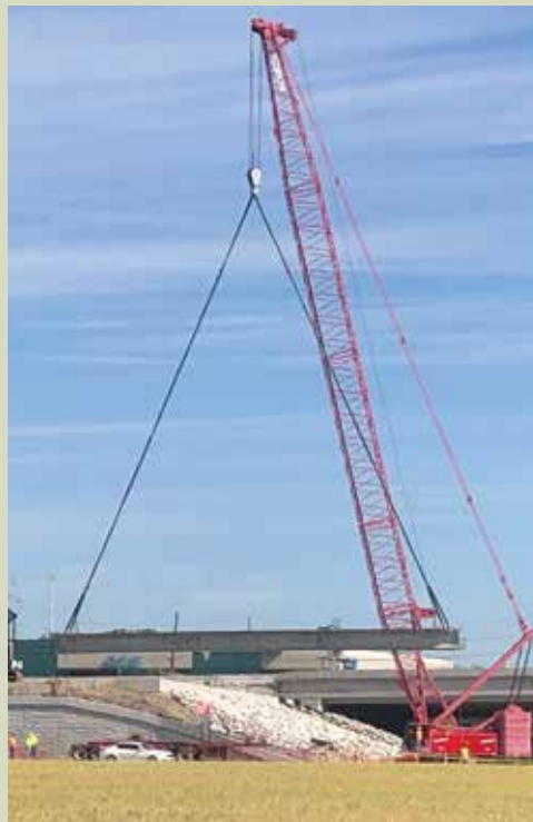
Mike Hardt and Kolton Goldsmith setting the first precast beams on the south bridge at Hwy 44 & the Meramec River for KCI. It's a MODot project.
