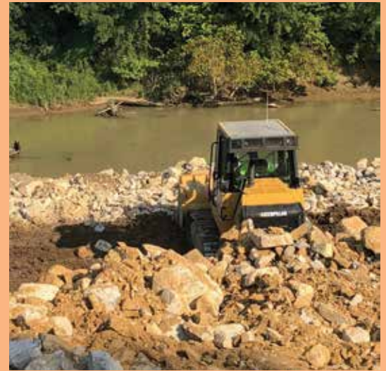
Charlie Picou working for Bloomsdale Excavating on the Diversion Channel Job outside of Delta, Mo.
