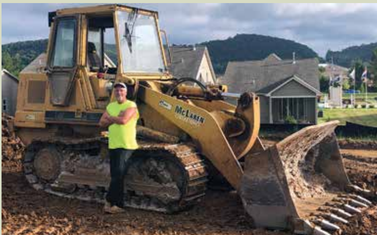
Richard Johnson working for L.S.M. Grading at the Windswept Farms subdivision in Eureka, a McBride Homes project.
