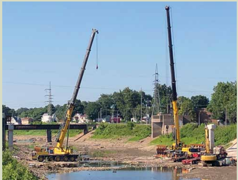
John Ramsey, Josh Hadler, Andrew Eye, David Branch and Joe Keith. All working for Taylor Excavating setting the pedestrian bridge on the Greenway Trail Project for Gershenson along Hwy. 55 and River DesPeres.
