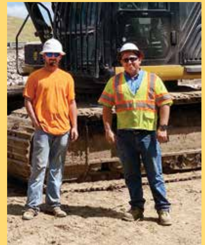
Premier Demolition - Tearing down the 18th St. bridge making way for the new MLS Soccer Stadium exit and entrance ramps - Austin Miller and Josh Kueker.
