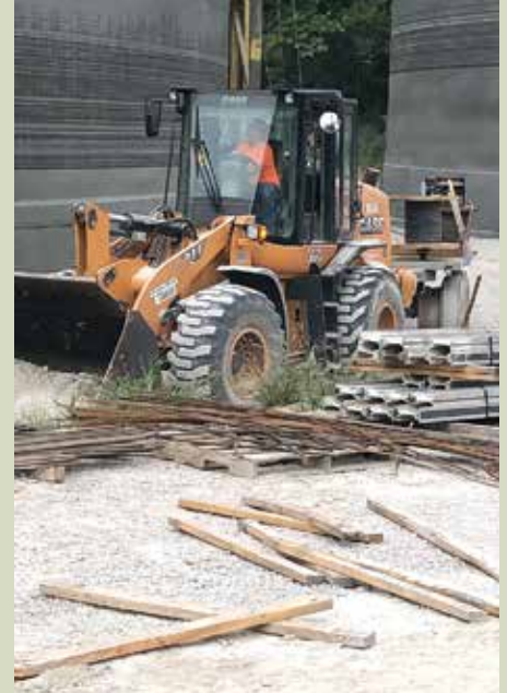
Dawn Mencin working for DN Tanks, a MSD Clean Stream project. Plocher Construction is general.
