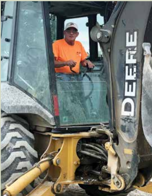
Shawn Null working for Lamke 'Trenching & Excavating digging the elevator shaft on the new entrance at the Hixson Middle School, a Jacobsmeyer Construction project.
