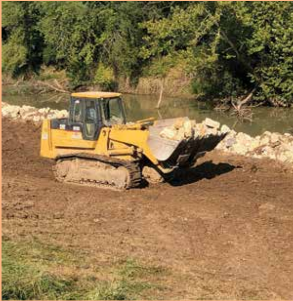
Kelly Christisen working for Bloomsdale Excavating on the Diversion Channel Job outside of Delta, Mo.
