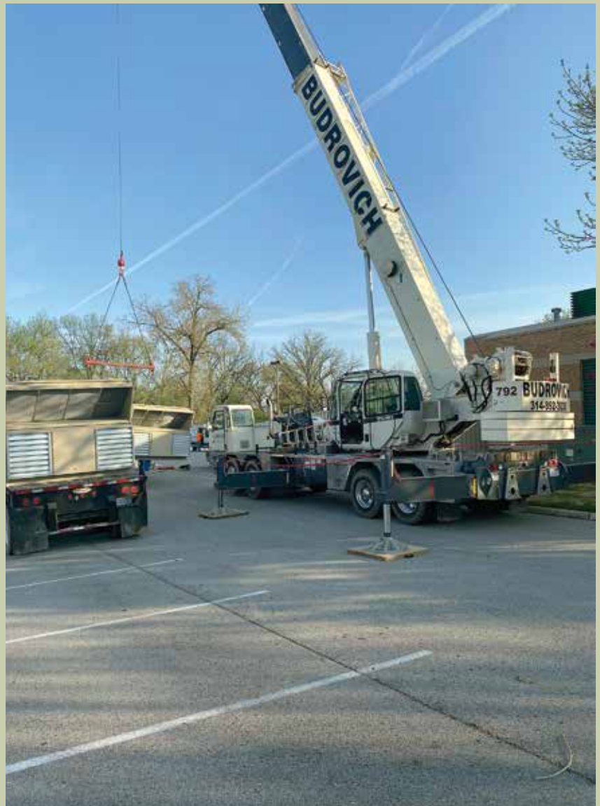
Steve Leslie, Operator on Truck Crane setting A/C units. Tim Ott on Truck Hauling new units at the St. Louis Union Hall.
