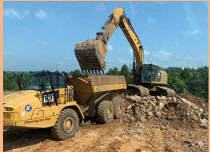
Jake Davidson in the 352 Cat Excavator and Scott Parsley in the articulated dump truck doing site remediation at the Cobalt Mine in Madison country.
