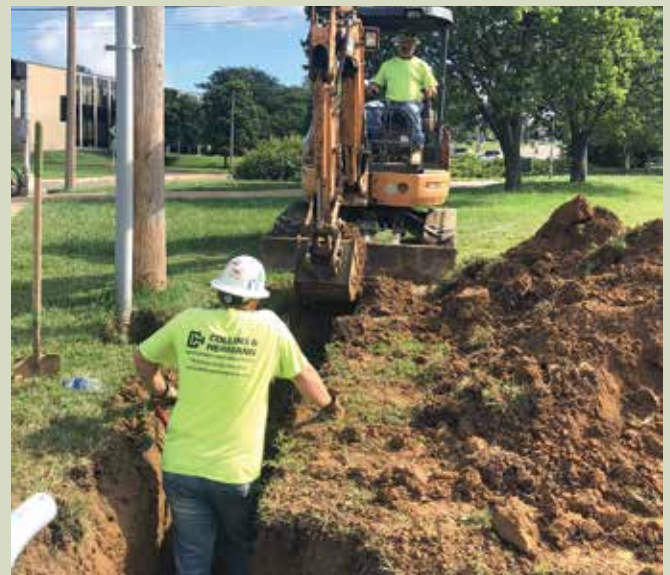
Michael Weirich working for Collins & Hermann on the utility work for the MSD Clean Stream tank project for Plocher Construction.
