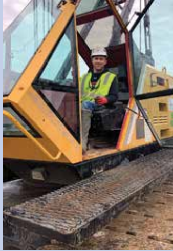
David Sparks assembling a crane for Phillips Hardy at Loure River on Hwy 70.
