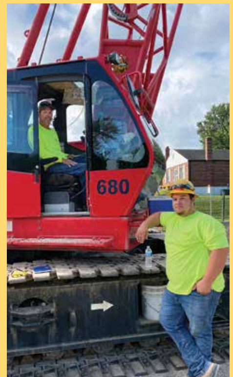
Goodwin Bros at the MSD Lower Maline Creek Project; Operator- Kenny Drury and Oiler -Luke Guzman.
