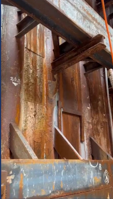
Significant water seepage → Action Level 2
