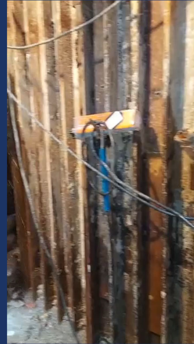
Excessive water ingress → Action Level 3
