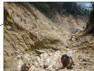
Eroded flow path
