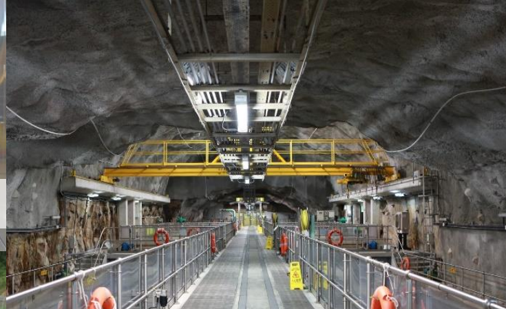
Stanley Sewage Treatment Works (1995)
