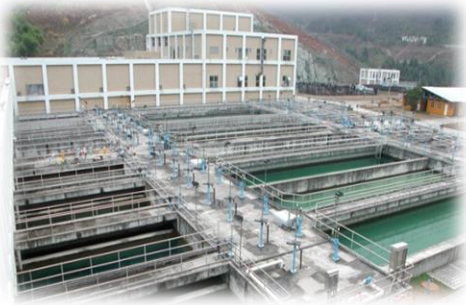
Sewage treatment works
