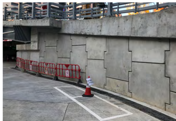
Figure 4j: Completion of Reinforced Earth wall with L-shape R.C. seating with steel girder ramp erected
