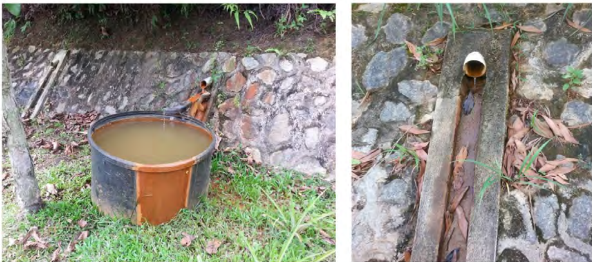
Plate 1: Continuous discharge of groundwater from the horizontal drains on site
