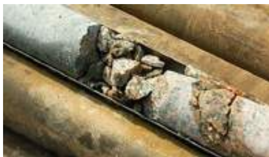
(a) Bentonite on Concrete Face, Concrete and Rock Fragments, and Core Loss
