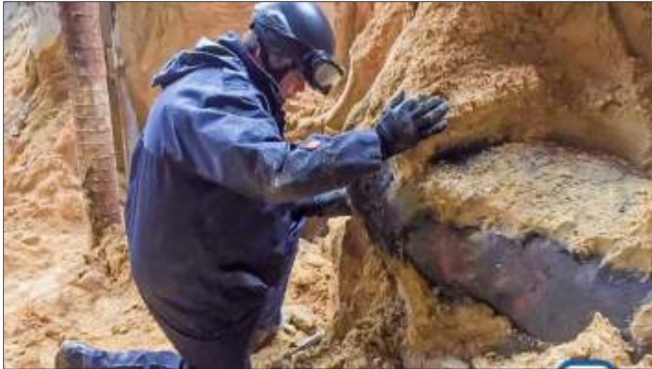
Figure 1: One of two WW2 x 1,000 lb AN-M65 bombs discovered on a waterfront construction site. January 2018, Convention Avenue, Wanchai (courtesy South China Morning Post)
