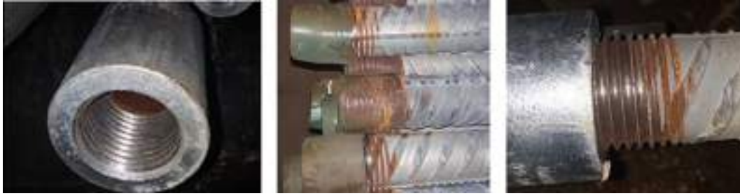
Plate 5: Machined thread, left: Black thread within a machined HDG coupler, middle/right: Machined threaded bar with uncorroded and corroded thread ends of HDG re-bars (DYWIDAG Archive)
