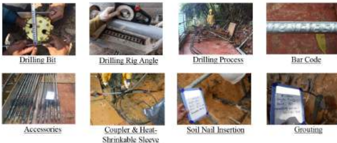
Plate 1: Examples of record photographs taken for each step of soil nail installation
