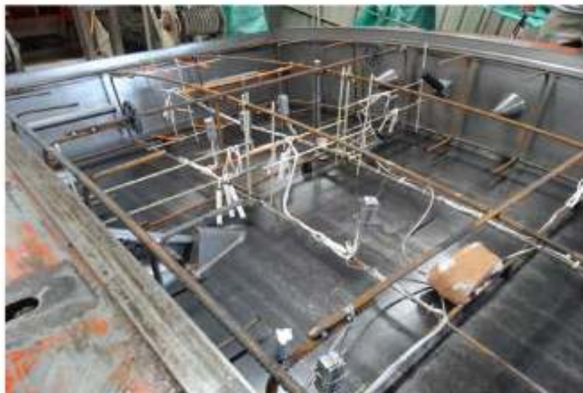
Figure 7: Instruments mounted in-situ; 80% less wiring than VW methods
