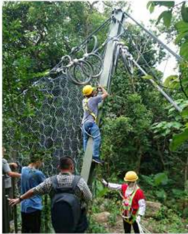
Plate 3: Photograph Showing the Repositioning of the T&V Sensor
