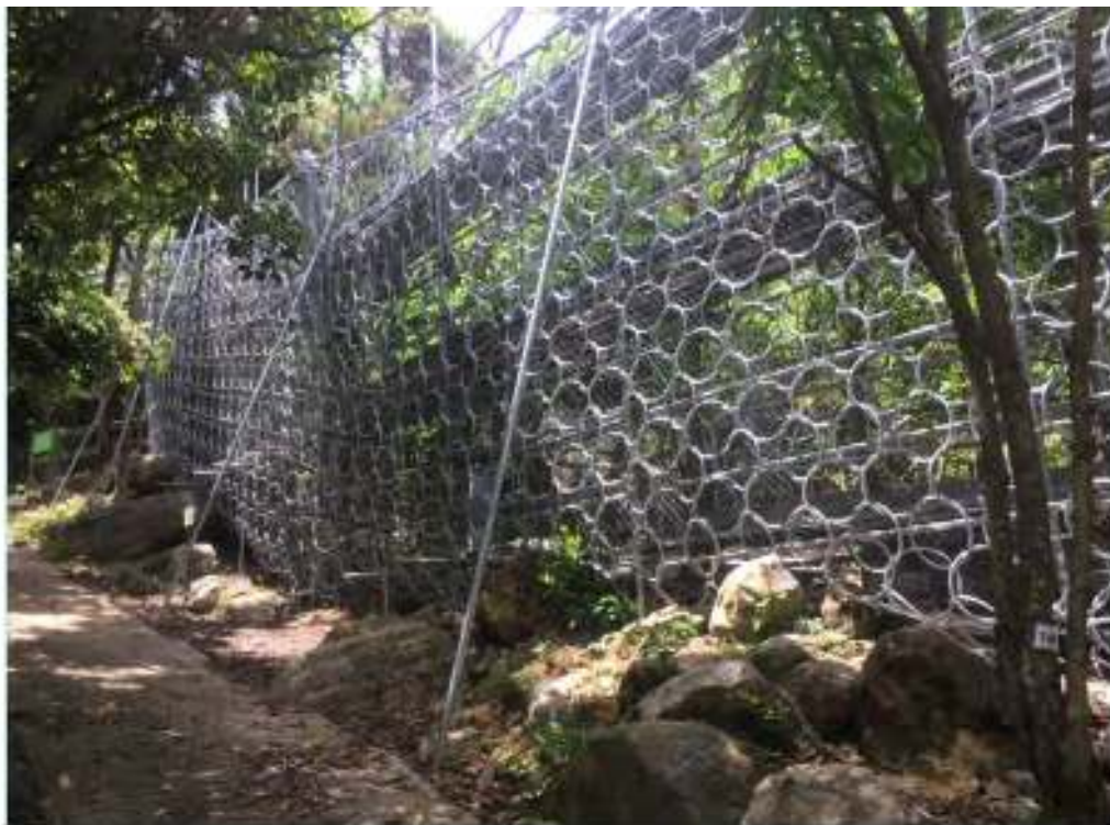
Plate 1: Typical Flexible Barrier in Hong Kong
