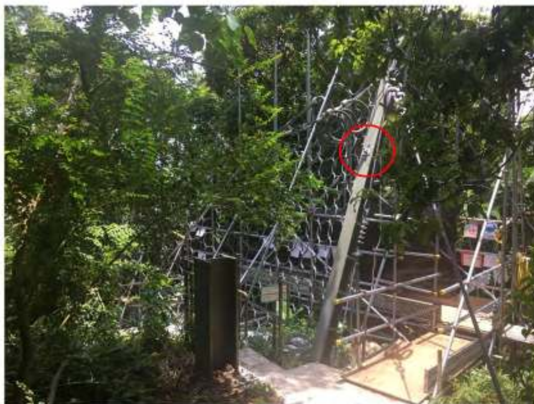
Plate 2: Wireless Tilt & Vibration Sensor Installed on the Steel Post
