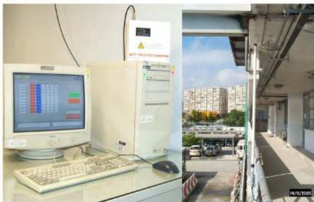
Plate 3: Cable free radio logger and antenna setup
