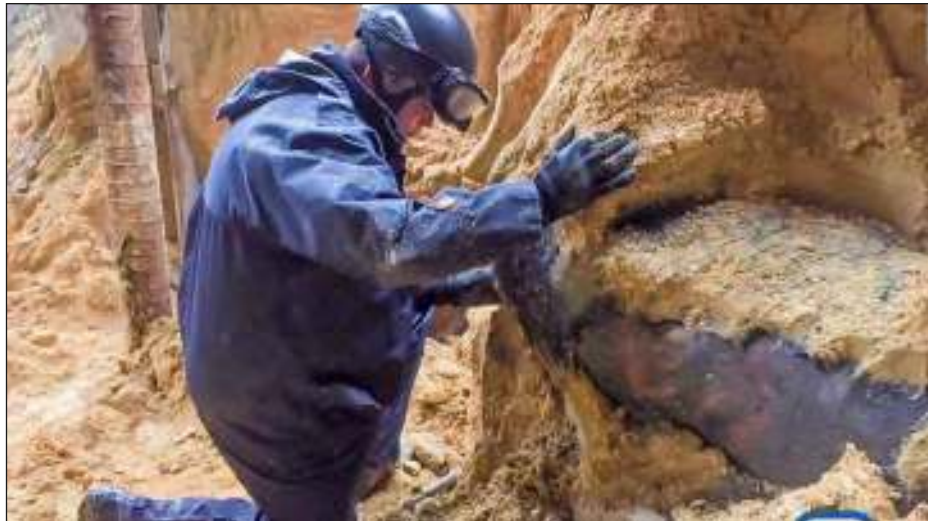
Plate 1: One of two 1,000 lb bombs uncovered at a construction site in Wan Chai North in January 2018. (South China Morning Post, 2018)
