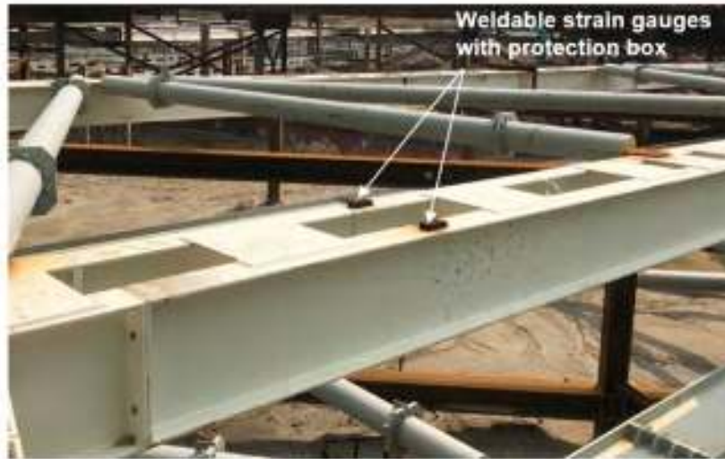
Plate 9: Wireless monitoring sensors
