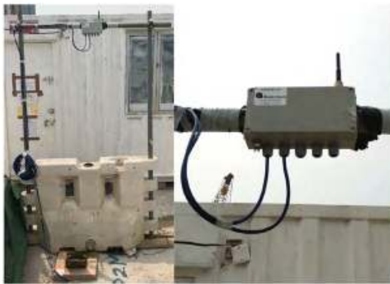
Plate 7: Ground water level monitoring using Loadsensing LS-G6-VW node
