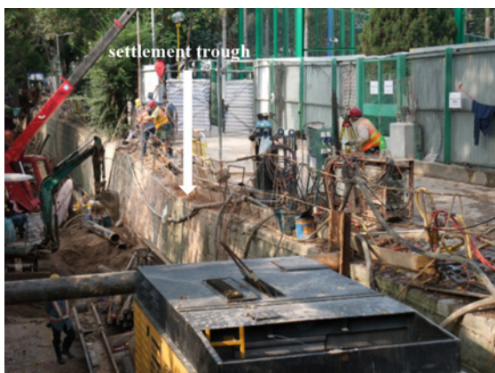
Plate 2: Settlement caused by Odex drilling
