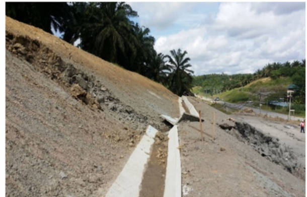
Figure 8: Side view of slope failure in highly and slightly weathered mudstones at Case 3
