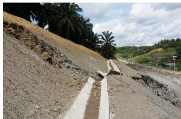
Figure 8: Side view of slope failure in highly and slightly weathered mudstones at Case 3
