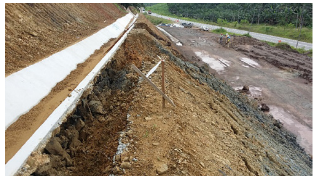
Figure 11: Side view of the slope failure at Case 4. The guiding frame on the sliding block is vertical.
