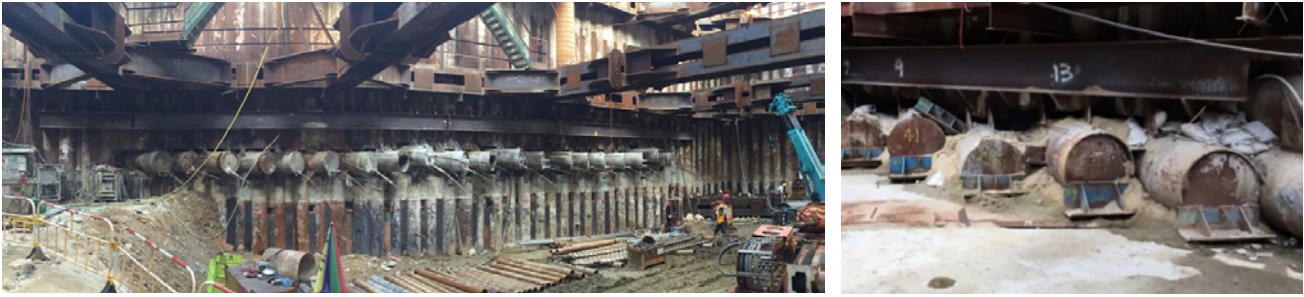
Figure 7(a): Installed Canopies from Launch Shaft to Receiving Shaft (b): Canopy Tubes Supported By Tunnel Box
