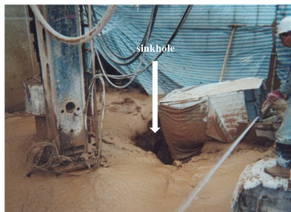
Plate 3: Sinkhole caused by Odex drilling
