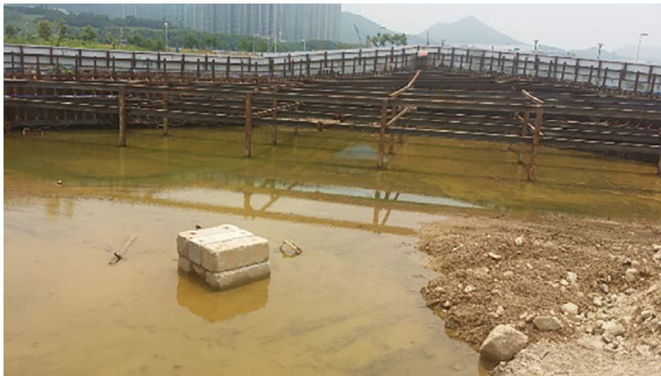
Plate 1: Photograph of a flooded cofferdam caused by leakage through pipe piles
