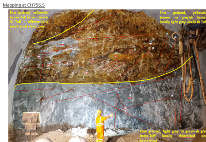
Figure 6 – Condition of tunnel face at CH756.5 showing a differentially weathered weak zone clearly defined and locally chloritized and brecciated tuff
