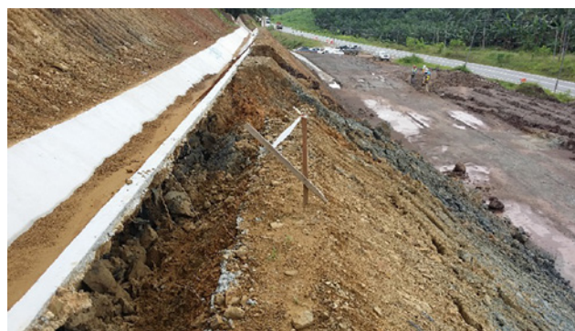
Figure 11: Side view of the slope failure at Case 4. The guiding frame on the sliding block is vertical.
