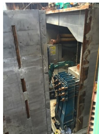
Figure 14: Side Wall of T002 Showing Lubrication Channels and Skirt Plates
