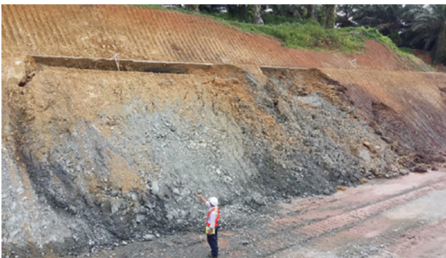
Figure 10: Front view of slope failure in slightly weathered mudstone for Case 4
