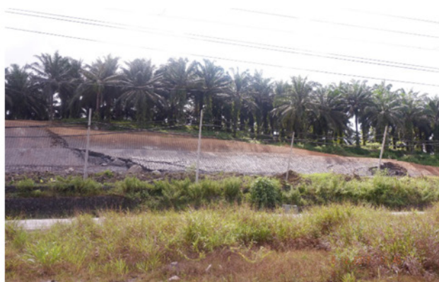
Figure 7: Front view of slope failure in highly and slightly weathered mudstone at Case 3
