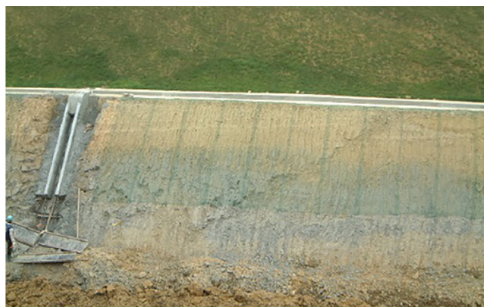
Figure 4: Pre-failure slope at Case 1 showing the joint plane intersecting the slope surface
