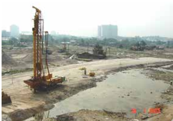
Figure 12: Stone columns being installed over soft, water-logged soils from a stable working platform.
