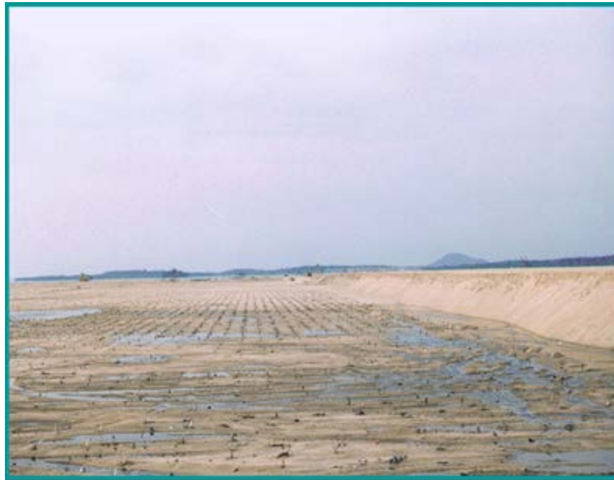
Plate 4: Large scale installation of flexible drains (Photograph courtesy of Prof J Chu)
