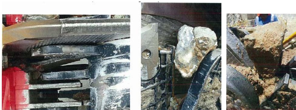
Plate 4: Hard rocks blocked at cutter plates found in trial panels
