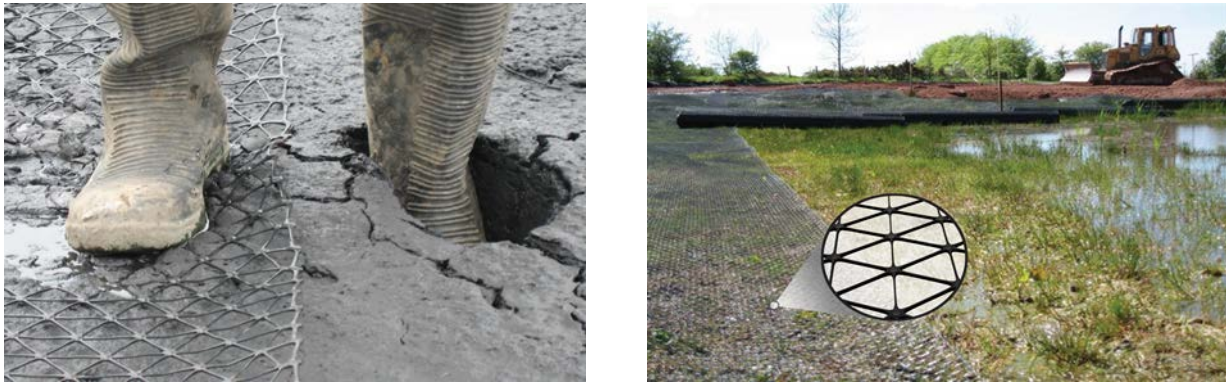
Figure 4: Two examples of ground stabilisation using hexagonal geogrids over extremely soft soils
