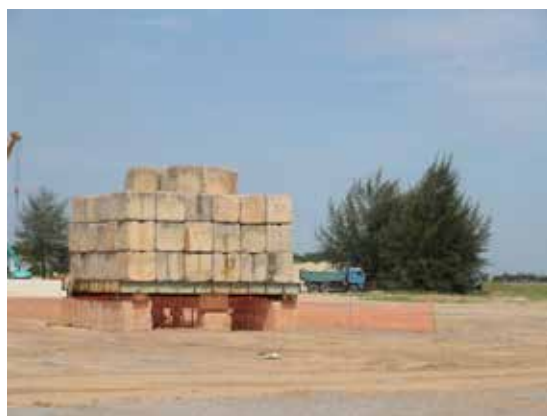
Figure 8: 175-ton kentledge load test on a single column using a 2.3 m x 2.3 m plate (Singapore, 2005)
