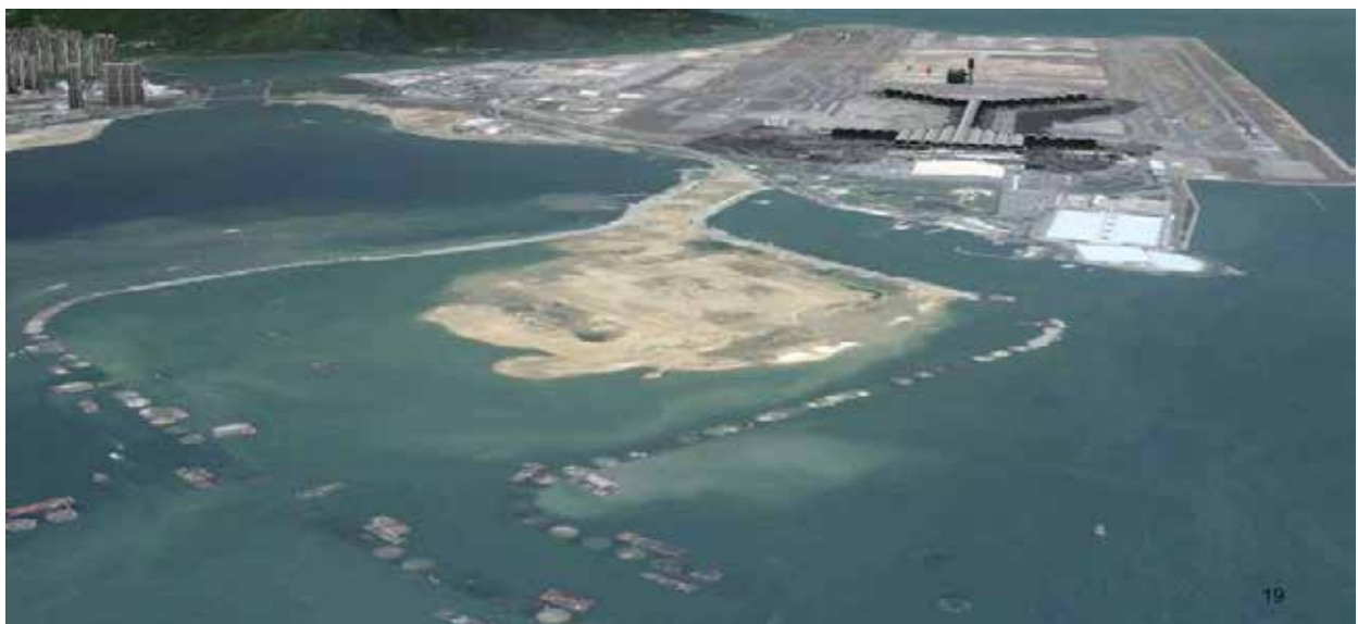
Figure 19: Outline of the steel cells installation formed as part of the seawall construction (April, 2014)
