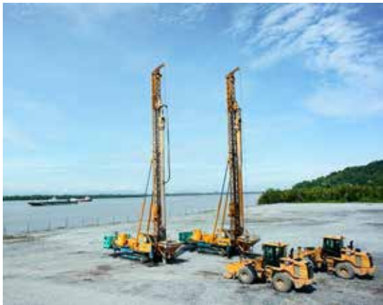
Figure 3: Dry bottom-feed columns installed for a dockyard, using purpose-built rigs (East Malaysia, 2014)
