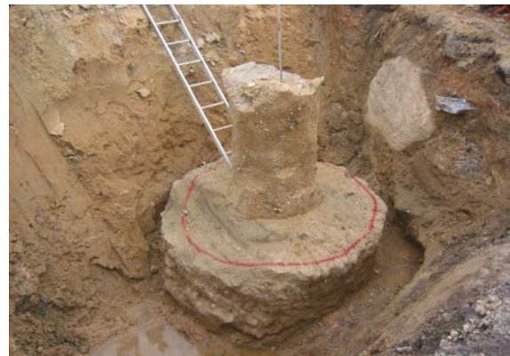
Figure 4: Exposed jet grout column A2
