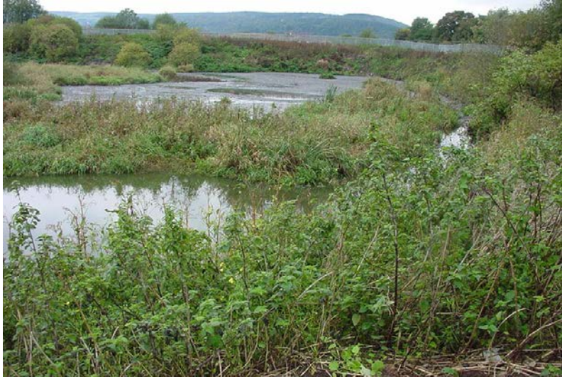
Figure 10: Sludge lagoon at Dowley Gap STW required capping
