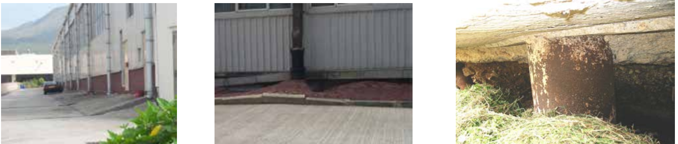
Figure 1: Damage caused by on-going post reclamation settlement
