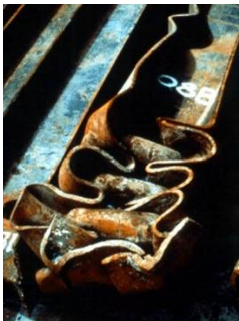
(a) Tip buckling of H-pile
