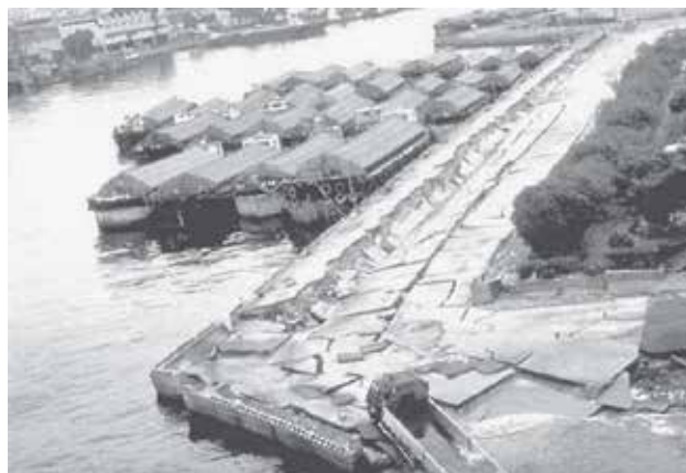
Figure 2: Retaining wall damage caused by liquefaction in the Kobe earthquake in 1995 (Photograph from the Kobe Geotechnical Collection, EERC, University of California, Berkeley)
