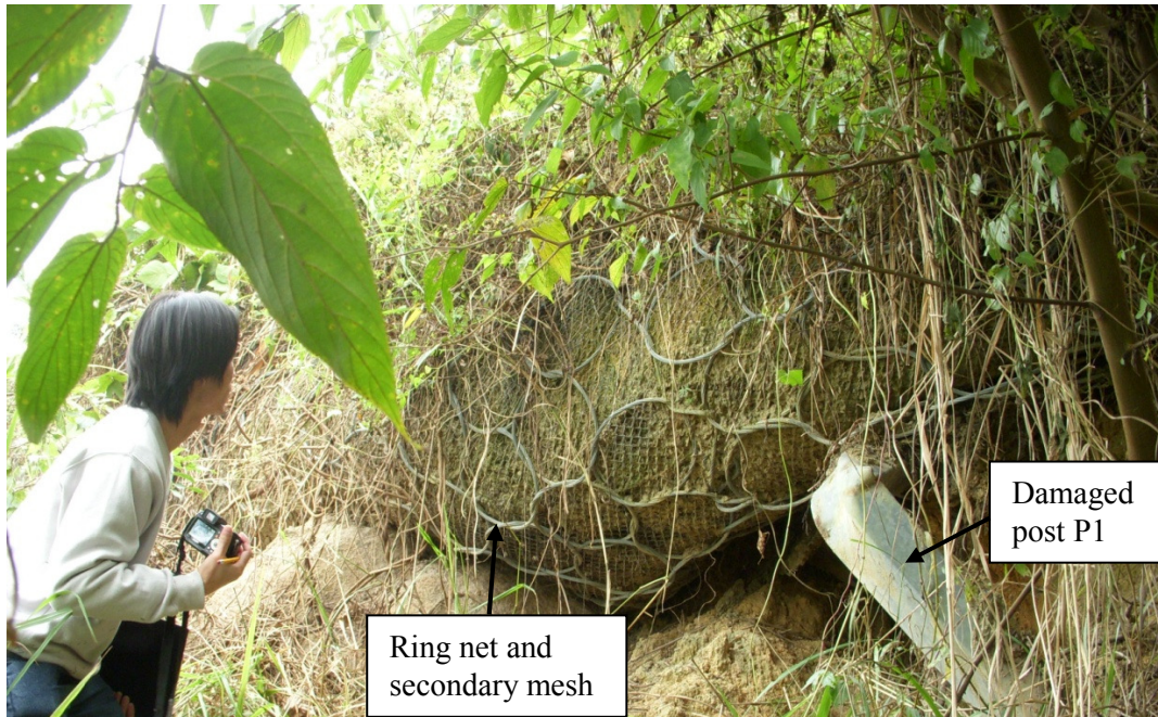
Figure 2: Landslide Debris Intercepted by a Flexible Barrier at Jordan Valley, Hong Kong (Kwan et al. 2014)
