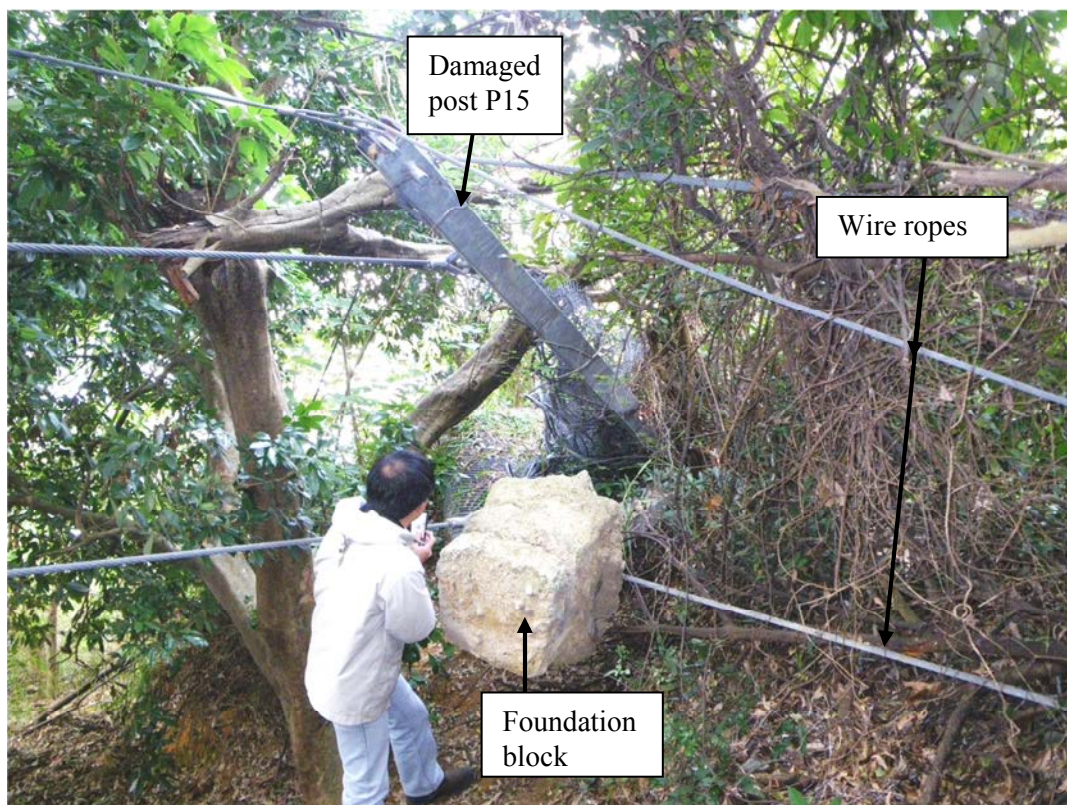
Figure 3: The Damaged Steel Post P15 and Its Uplifted Foundation Block
