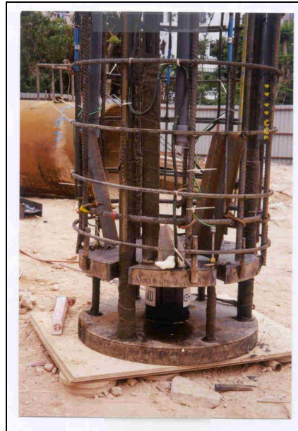
Figure 5B – Assembled jacking device attached to the bottom of reinforcing steel cage
