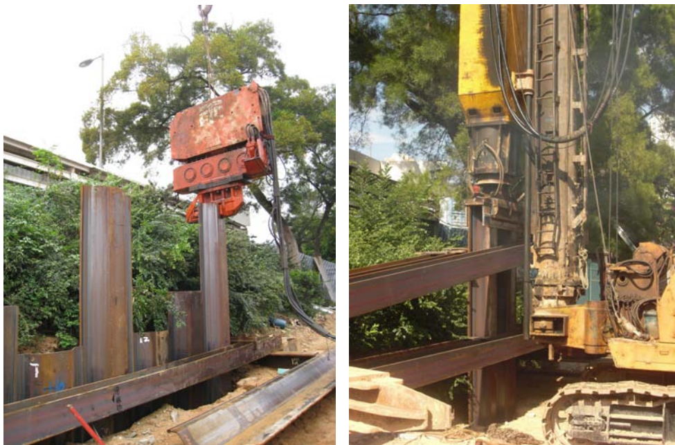
Figure 6: Installation of Hat-type sheetpile by vibratory hammer (left) and hydraulic hammer (right) at Site B
