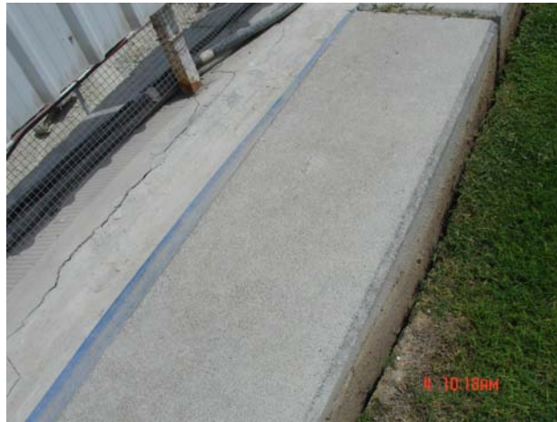
Plate 2: Ground depression behind secant pile wall
