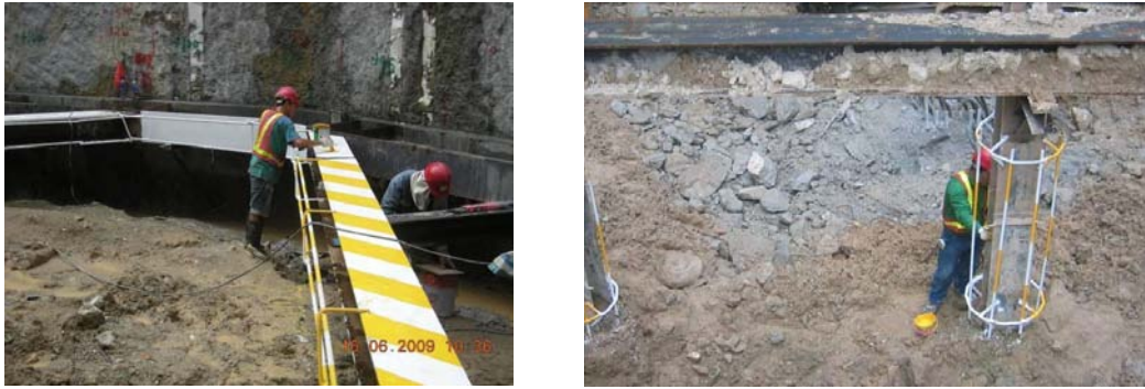
Figure 6: Strut and waling (left) and king post (right) protected by anti-collision rebars
