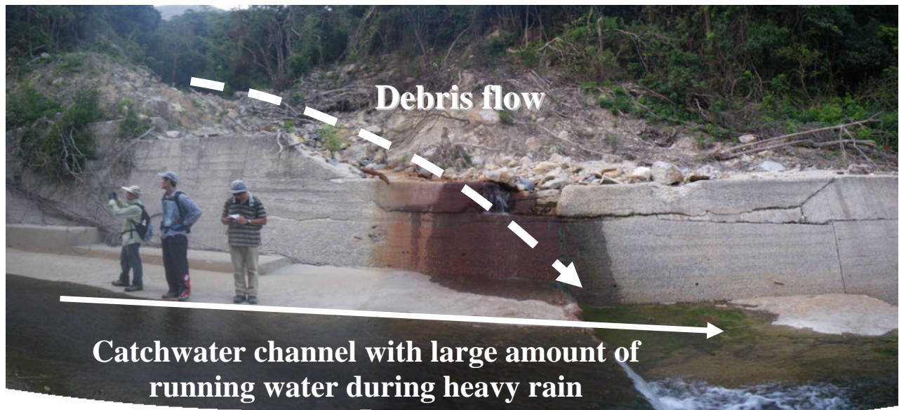
Figure 37: Debris flow entering catchwater channel (Note: The June 2008 Shek Pik No. 1 debris flow is shown; the debris flow turned into a debris flood after entering the catchwater channel)
