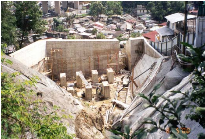
(a) Single debris-resisting barrier at the toe of drainage line
