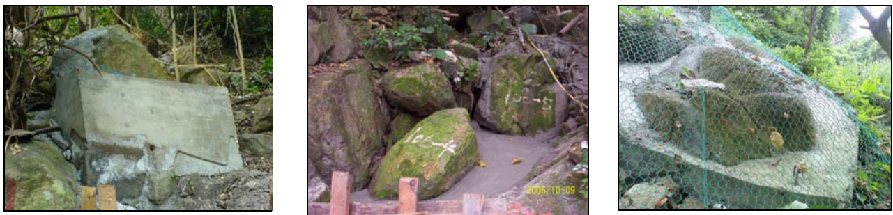
Plate 6: Preventive mitigation measures (in situ stabilization of boulders – buttressing, concrete matrix and wire meshing)
