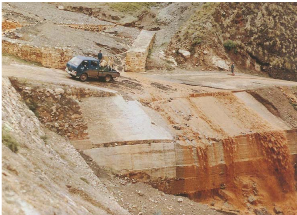
Figure 9: Overflow pavement is a feasible scheme when a road must pass through debris flow field where the bridge and tunnel not be constructed for economic or technical reason. Although the overflow pavement is economical and easy to build, it should be located in stable section eroded and deposited by debris flow. The concrete overflow pavement in Wangjiaqing valley, Dongchuan, Yunnan Province, is located in the key area where the erosion and deposition of debris flow reached equilibrium and has resisted debris flow hazards for over 20 years
