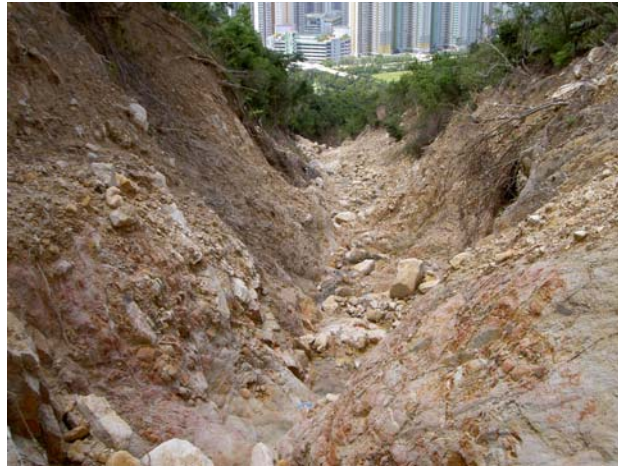
Figure 31: Complete removal of perched materials in the depletion zone of debris flow (Note: The June 2008 Yu Tung Road debris flow is shown; the side slopes and bed of the drainage lines not subject to significant material loss)
