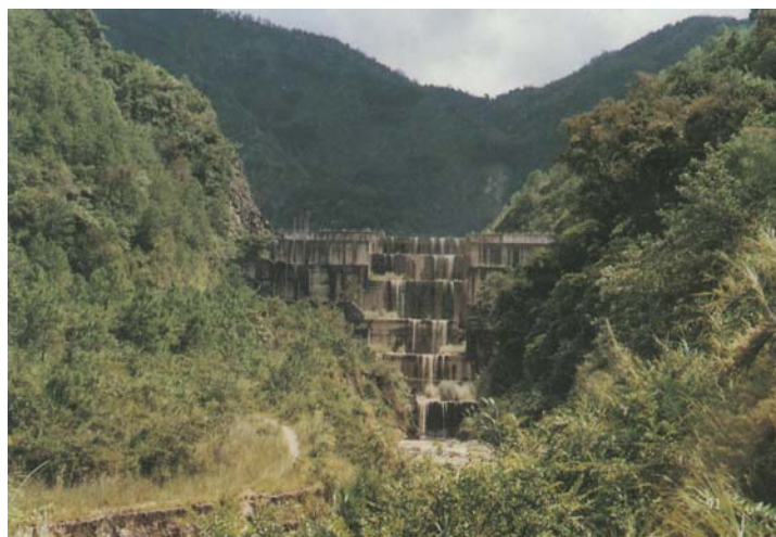
Figure 2: Hunshuigou valley step-dam is located in Yingjiang county, Yunnan province. It was constructed in 1998 and has deposited 6 million debris flow materials. It is 67 m (5 steps) and the highest debris flow storage sediment dam in the world by now.
