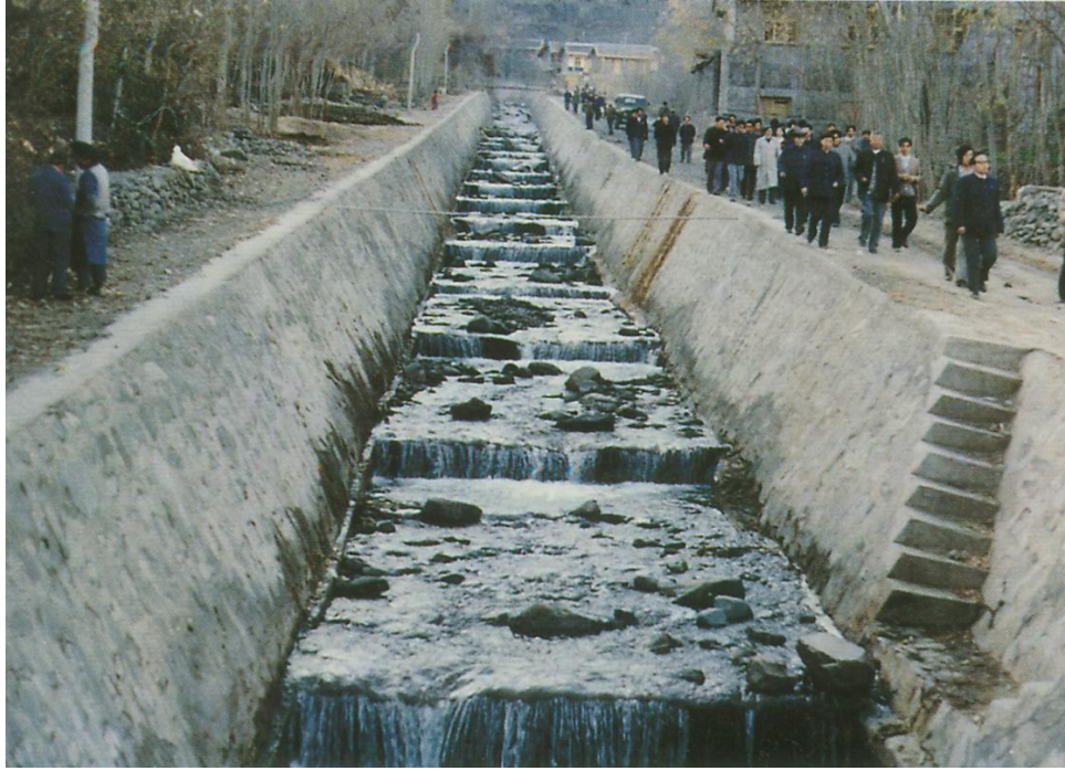
Figure 5: Babuligou valley drainage slot (to protect the city of Jinchuan county, Sichuan province)
