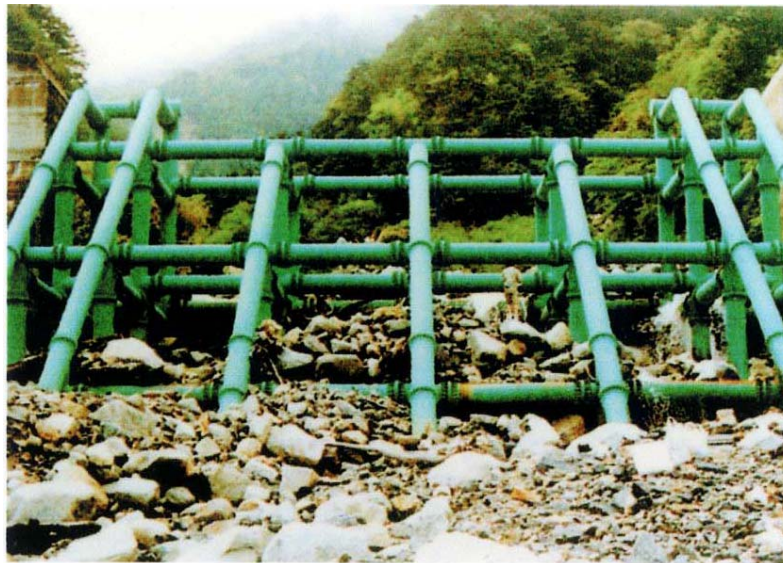
Figure 29: Grid-type steel sabo structure (Note: The open structure would trap sizeable clasts and allow free drainage; photo from Lo 2000)
