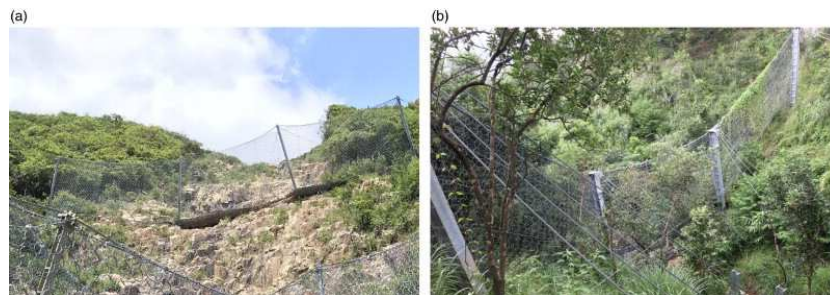
Figure 1. Examples of proprietary rockfall-resisting flexible barriers in Hong Kong installed: (a) on an open hillside; and (b) in an incised drainage line.
