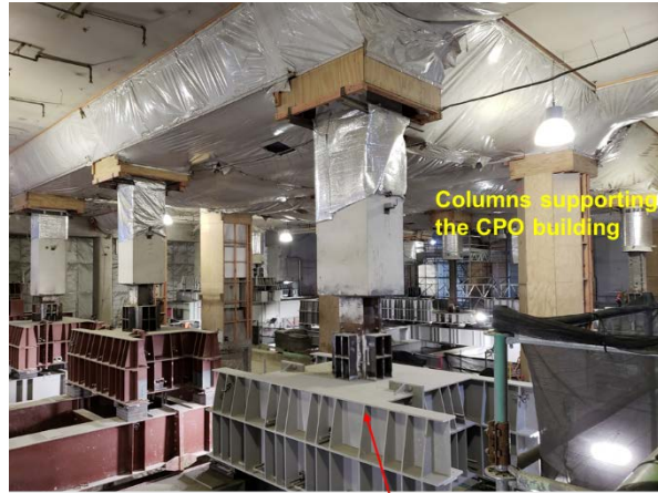
Hydraulic load cell and support frame
