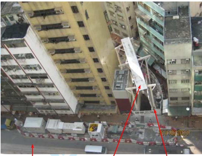
Des Voeux Road West 10 ton monorail gantry 51 dB(A) noise cover
