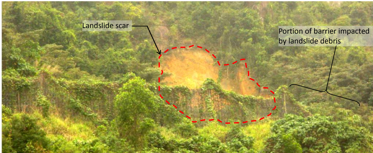
Figure 3 The landslide scar and the flexible rockfall barrier
