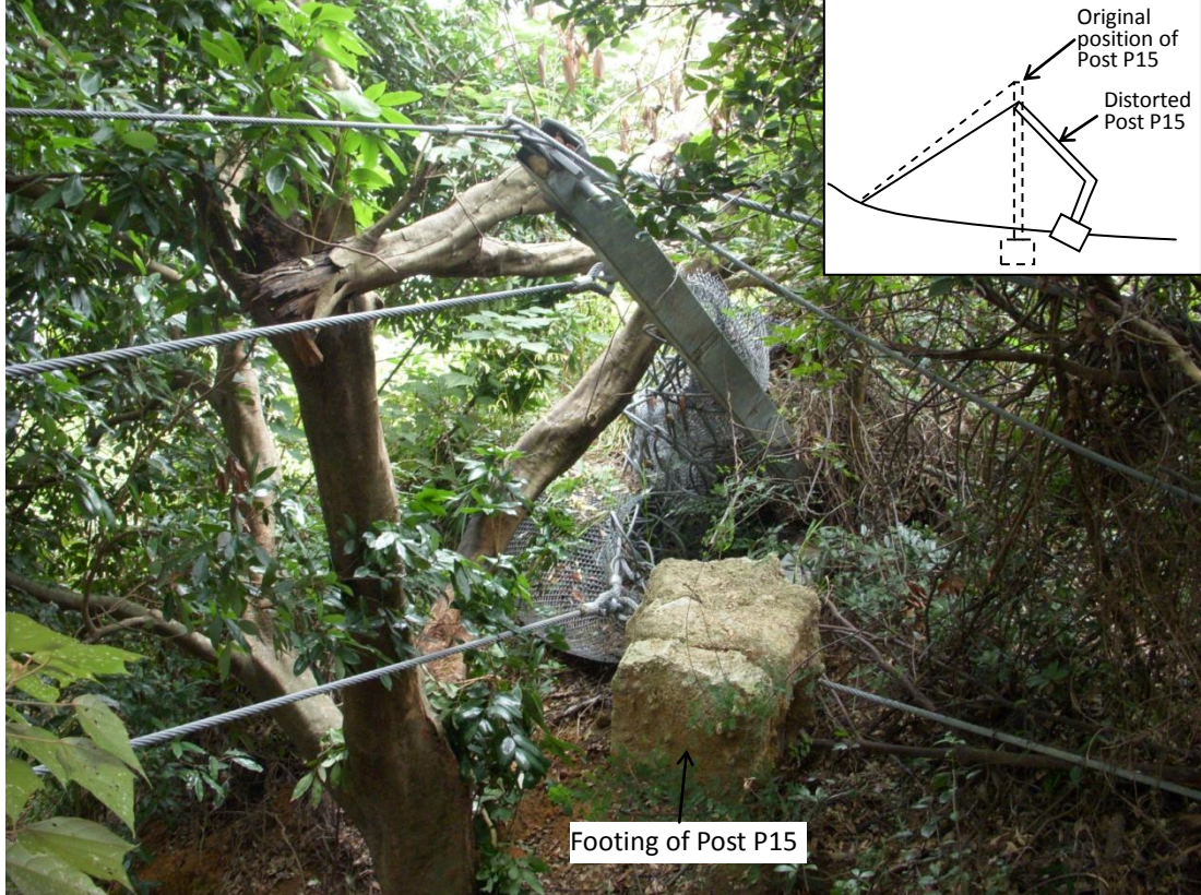
Figure 6 Post P15 severely bent and foundation failed
