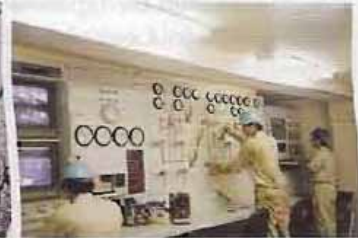
Picture.4 Control cabin for mixed-gas breathing system
