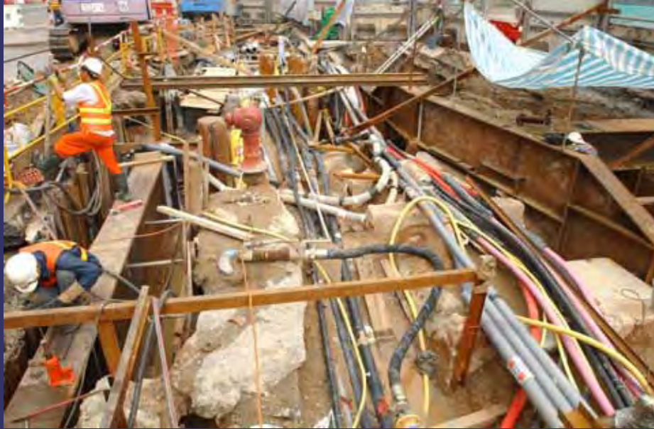
utilities & concrete surround obstructions
