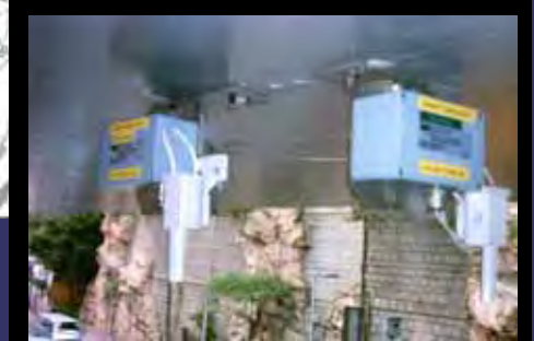
EL tilt sensors on bridge soffit
