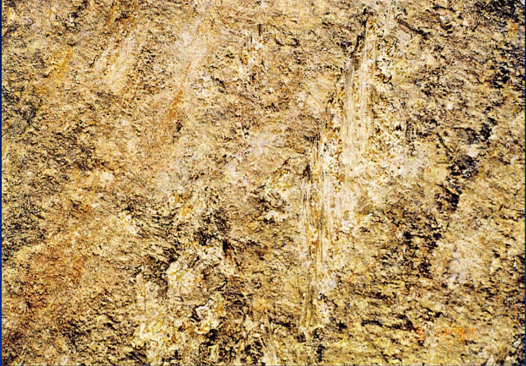
Slickensiding observed on the sub-vertical face of the largest block of rock
