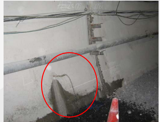
Detail: Water is behind the concrete shell!
